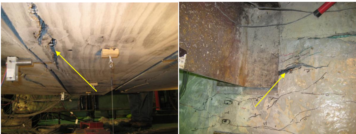
Figure 4.58. UHPC Rupture (Top and Bottom-of-Deck)
