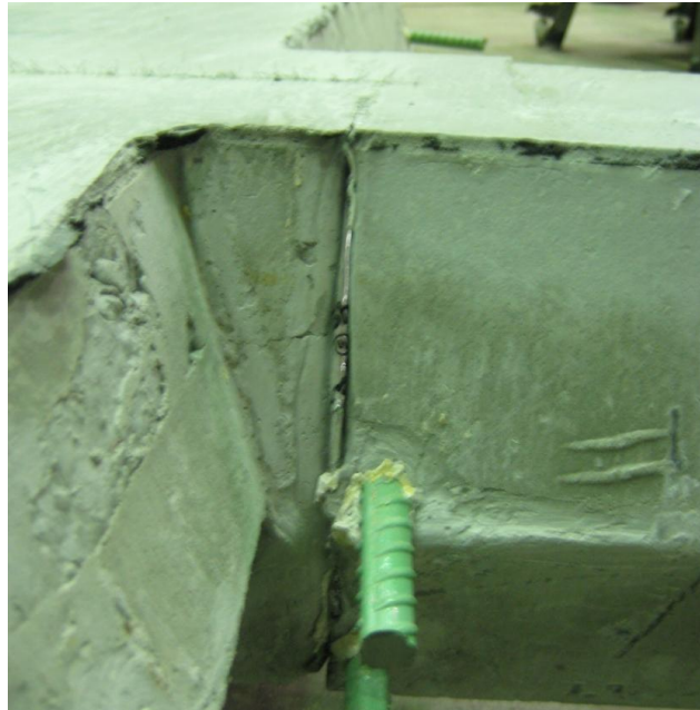
Figure 4.9. Stay-in-Place Acrylic Bulkhead
