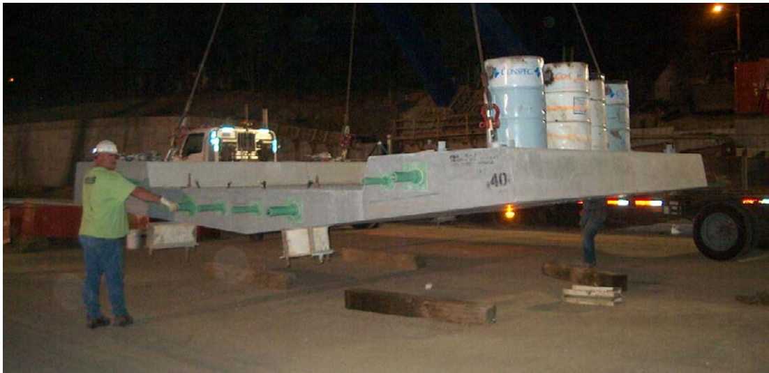
Figure 3.3. Sand-Filled Barrels Used as Ballast During the Erection of 40 th Street Bridge Panels
