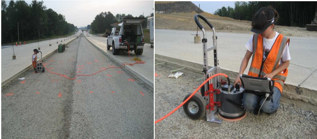
Figure 40. Overview for test bed (left) and GPT in situ testing on cement treated base on SR-22, Pennsylvania
