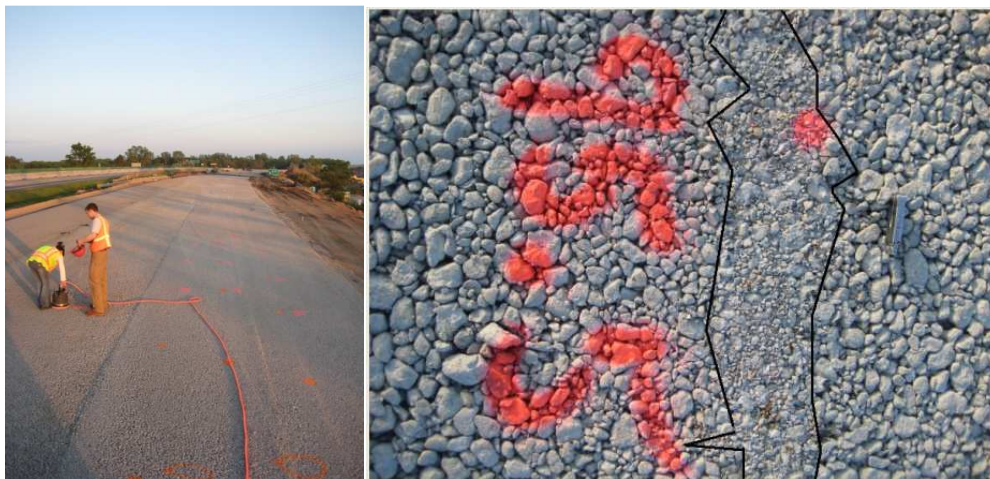
Figure 35. GPT on cement treated base (left) and segregation of CTB on I-96, Michigan.
