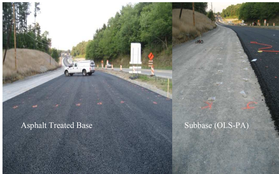
Figure 41. Overview for test bed (left) and subbase test location asphalt treated base on US-22, Pennsylvania
