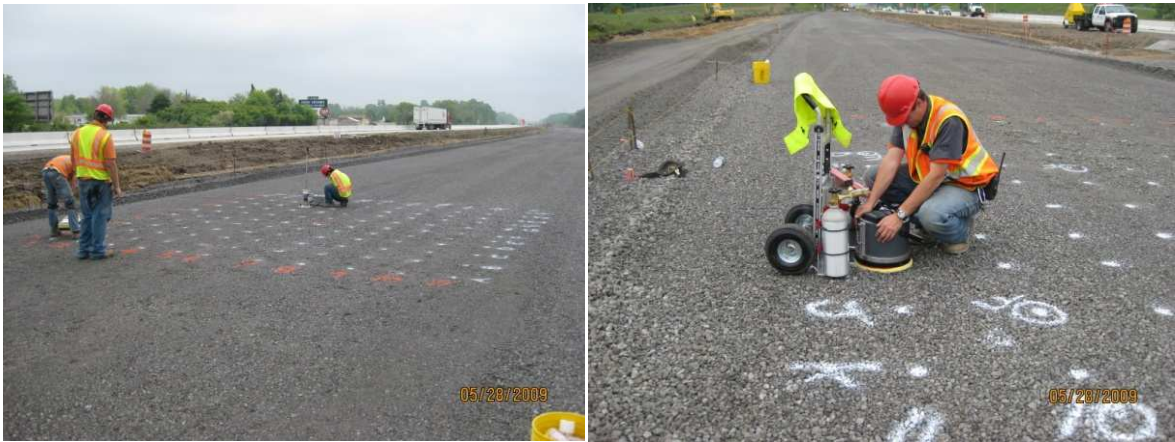
Figure 31. Overview for test bed (left) and GPT in situ testing on I-94, Michigan
