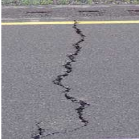
Figure 2.13 A Pictorial View of non-Load Associated Cracking (Low Temperature Cracking)
