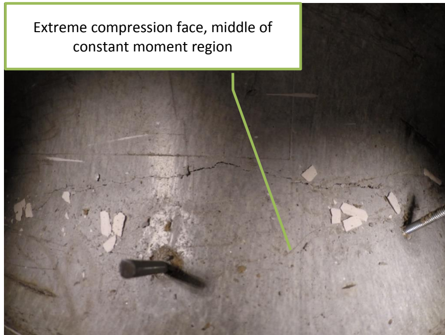
Figure 5-12: Inside Face of Specimen H2C2-C in Constant Moment Region under Compression
