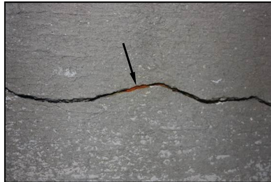
Figure 4.1 Rust observed at an intersection of steel with 2.5 mm-wide crack after continuously ponding in chloride for two weeks in specimen R12. (Indicated by arrow)
