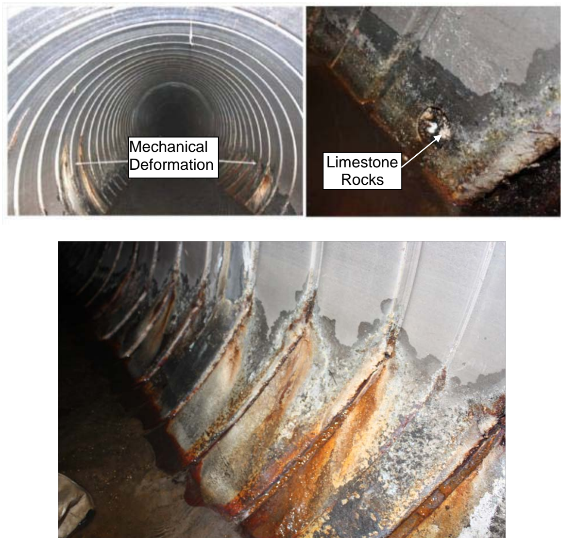
Figure 15: Photograph of in situ pipe located in Jacksonville, near Highland Glen and Beach Blvd. Mechanical damage (Top-left and bottom). Limestone rocks present beneath the bore location (Top-right).
