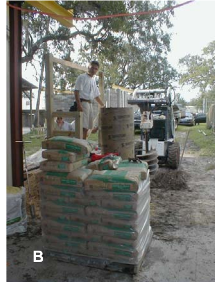
Figure 4.13 - Field trial #1 erected test shaft, A - top view of erected Sonotube, B - work platform and bags of type I cement
