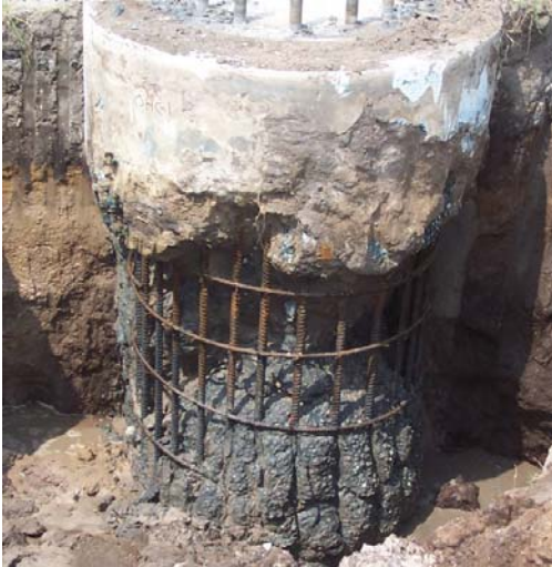
Figure 1.1 - Drilled shaft with absent concrete
