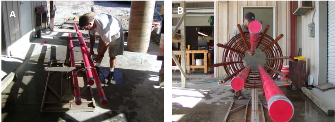
Figure 4.29 - Tying rebar cages for field trial #2, A - inclinometer casing and #3 ties, B - inclinometer casing and rebar cage for second shaft
