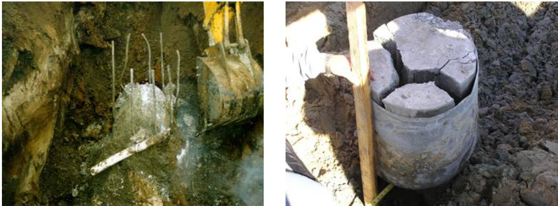
Figure 1.2 - Concrete failure at top of drilled shaft during load test (Left), concrete failure at top of drilled shaft during load test (Right) (Stokes, 2007)
