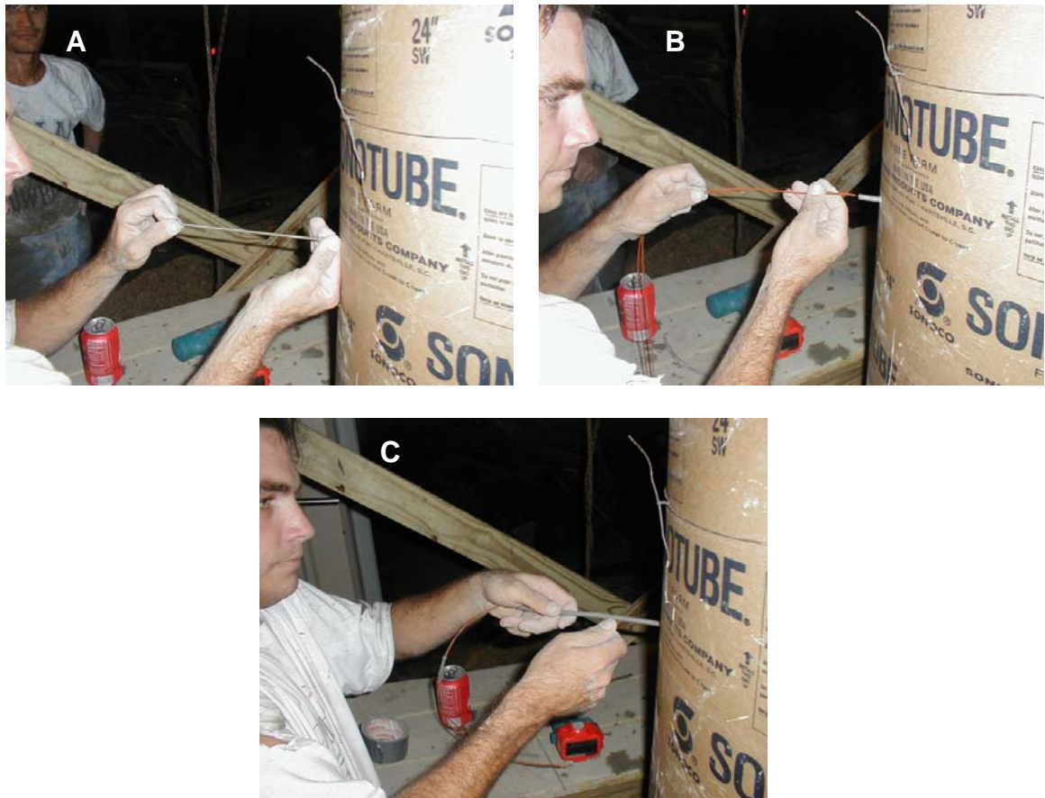
Figure 4.15 - Installing thermocouples in test shaft for field trial #1, A - inserting rubber tube into drilled shaft utilizing a welding rod, B - inserting two-wire thermocouples into capillary tube, C - removing capillary tube, leaving thermocouple in place
