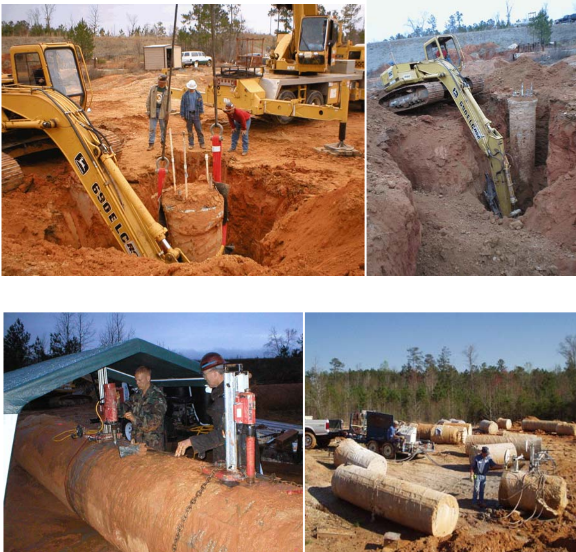
Figure 5.29 - Exhuming, coring and dissecting the test shafts at the Auburn test site
