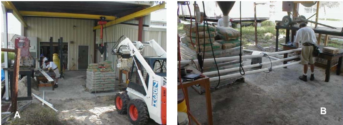
Figure 4.10 - Field trial #1 test set-up, A - location of test shaft, B -securing access tubes to #3 circular ties
