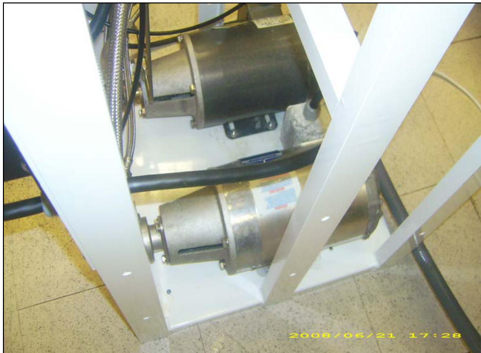
Figure 3-3. The assembled high pressure pump (top), and the permeate pump (bottom)
