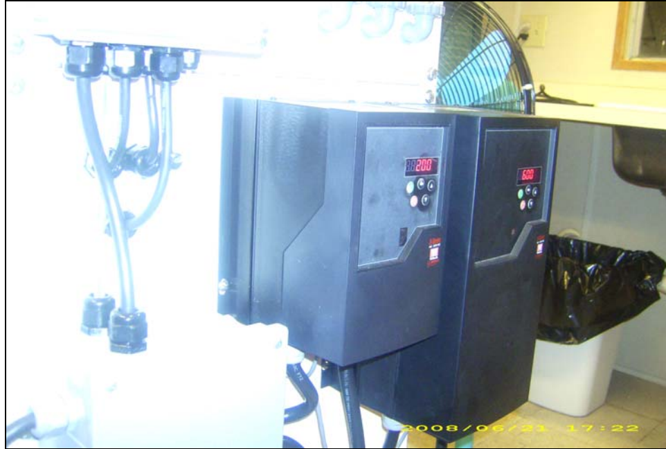
Figure 3-2. Variable frequency drives for the high pressure pump, and the permeate pump
