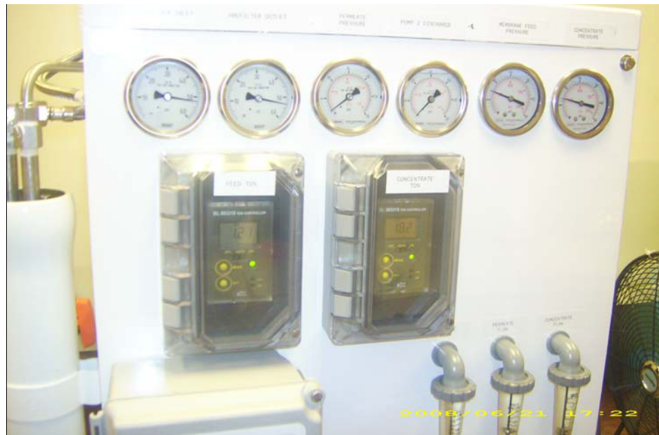
Figure 3-1. Experimental equipment skid showing pressure gauges, TDS meters, flowmeters, and NF membrane pressure vessel
