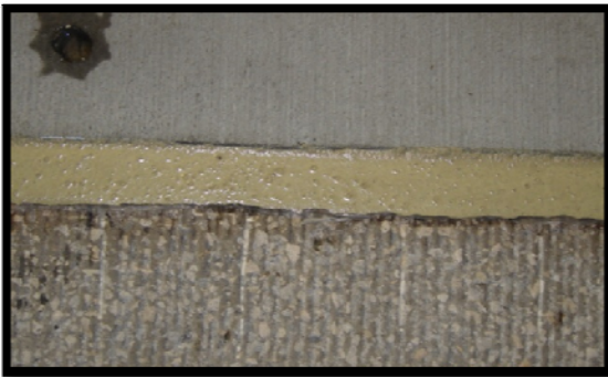
Figure 6.4 Installing Backer Rod for Pouring Epoxy and Finished Epoxy Joint for Bonding New Panel with Existing as well as Seating for New Panel
