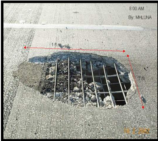
Figure B.2 Bridge No. 100332, Span 38- Asphalt Patch (Failure)
