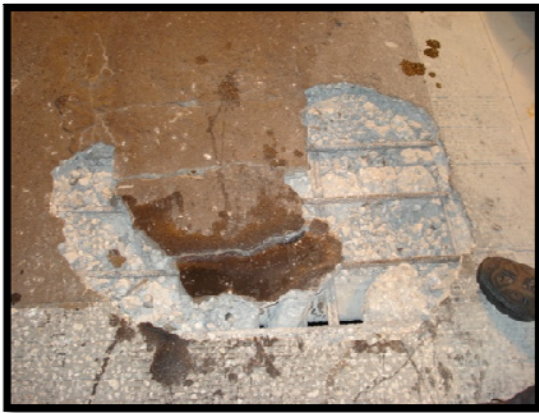
Figure 3.1 Bridge No. 100332, Span 39 Failure (Deck Top)
