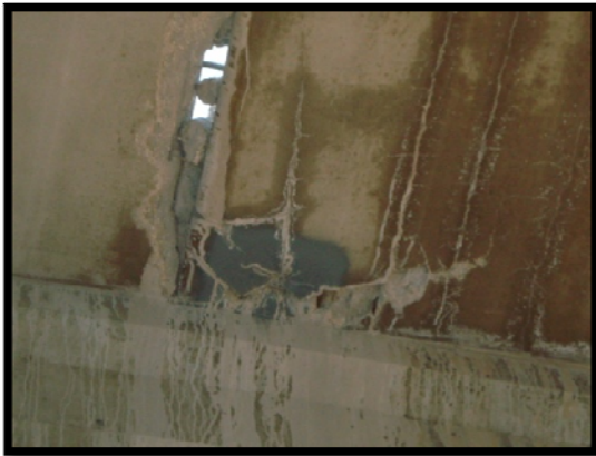
Figure 3.2 Bridge No. 100332, Span 39 Failure (Deck Underside)
