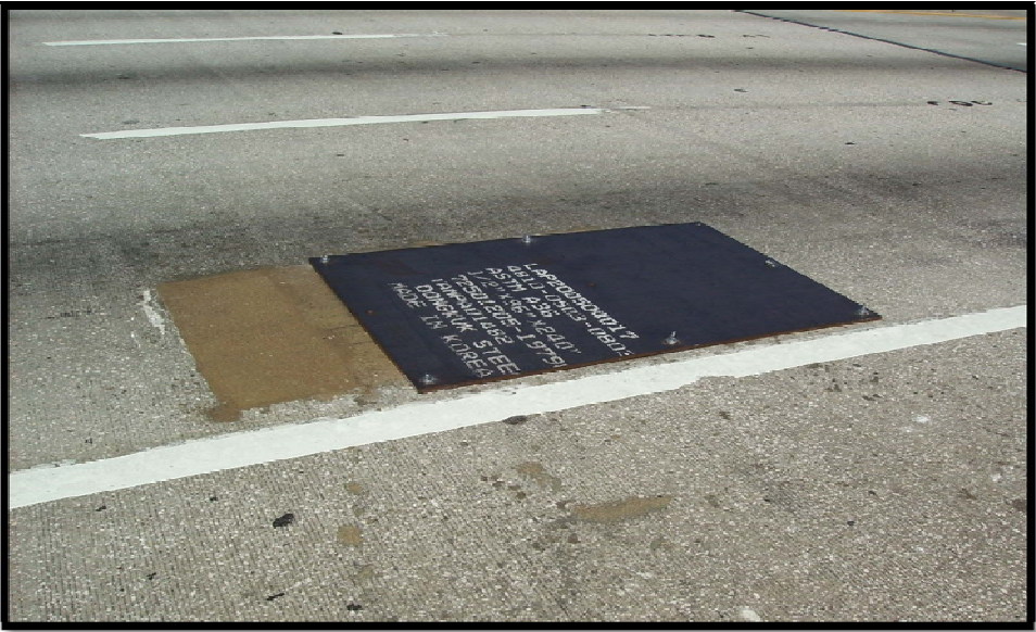
Figure 4.1 Bridge No. 100436, Span 4 Failure (Temporary Steel Plate)
