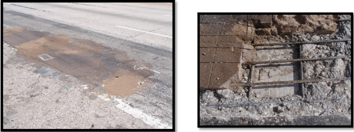
Figure 4.3 Bridge No. 100436, Span 4 (Failure in Patch Repair Material)
