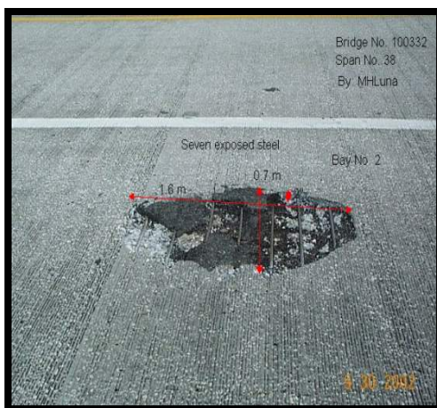
Figure B.1 Bridge No. 100332, Span 38- Asphalt Patch (2 Days Before Failure)
