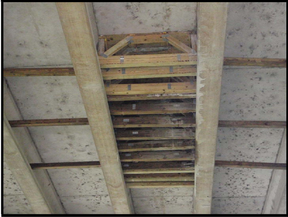
Figure 4.2 Bridge No. 100436, Span 4 Failure (Timber Bracing)
