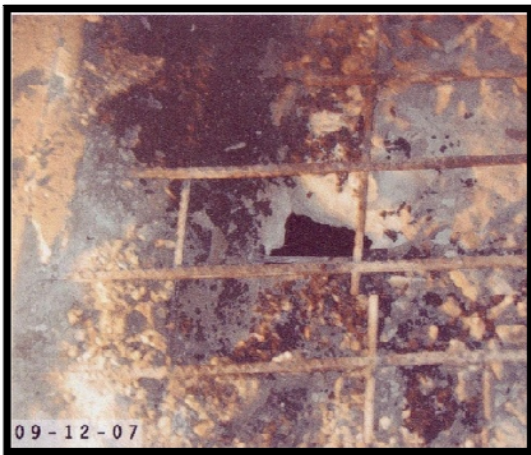
Figure 3.4 Bridge No. 100436, Span 4 Failure (Deck Top)
