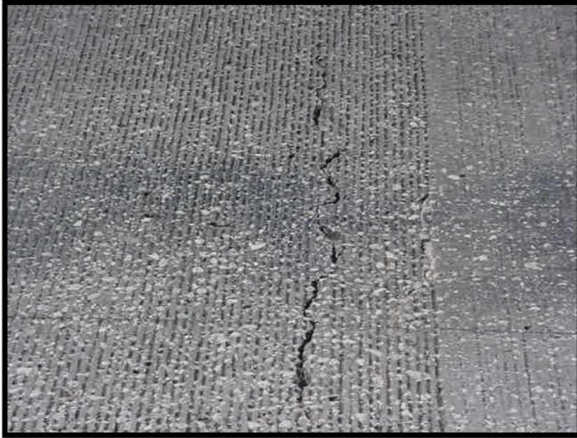
Figure 3.8 Bridge No. 100436, Span 4 Failure (3/4 in. Transverse Crack)
