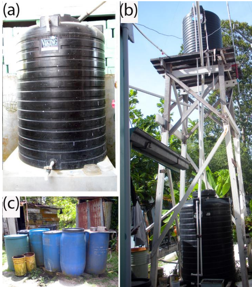
Figure 5.4 Representative water storage in Region 4 Subset, Guyana. (a) 450 gallon HDPE storage tank being filled with rainwater (roof runoff) from which water is collected at the base; (b) 450 gallon HDPE storage tanks on a trestle with the bottom tank collecting water from the main which is then pumped to the higher tank that then delivers water directly into the house; and (c) 55 gallon HDPE storage drums filled with water from a standpipe connected to the main.
