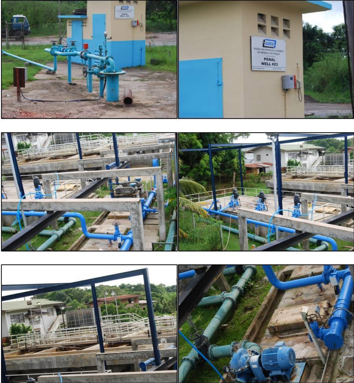
Figure D.4 Pictures from Water and Sewerage Authority of Trinidad and Tobago (WASA), Penal Plant.
