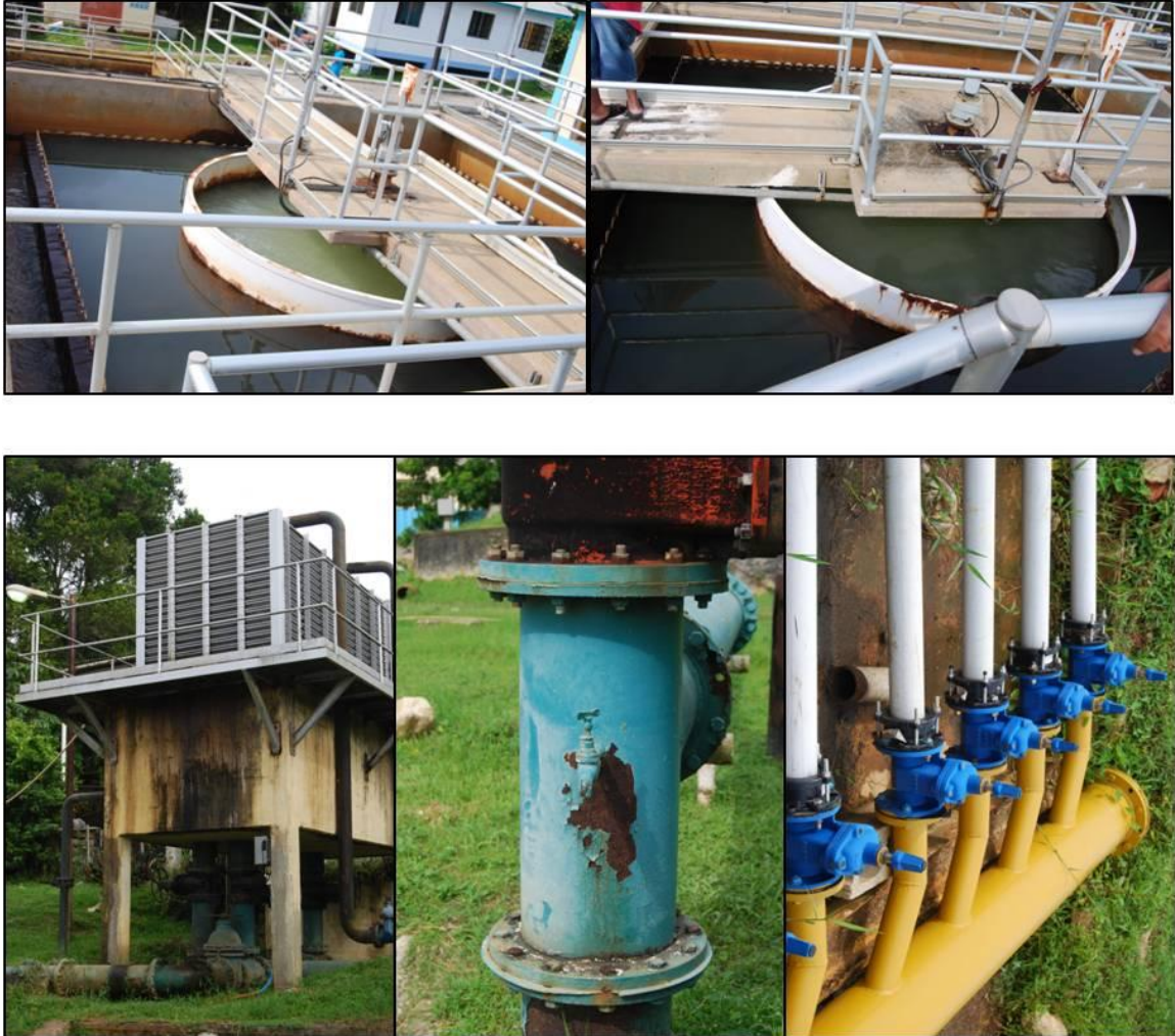
Figure D.5 Infrastructures at the Water and Sewerage Authority of Trinidad and Tobago (WASA), Penal Plant.
