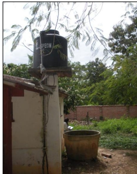
Figure D.16 Elevated black water storage tanks in Villa Litoral, Bolivia.
