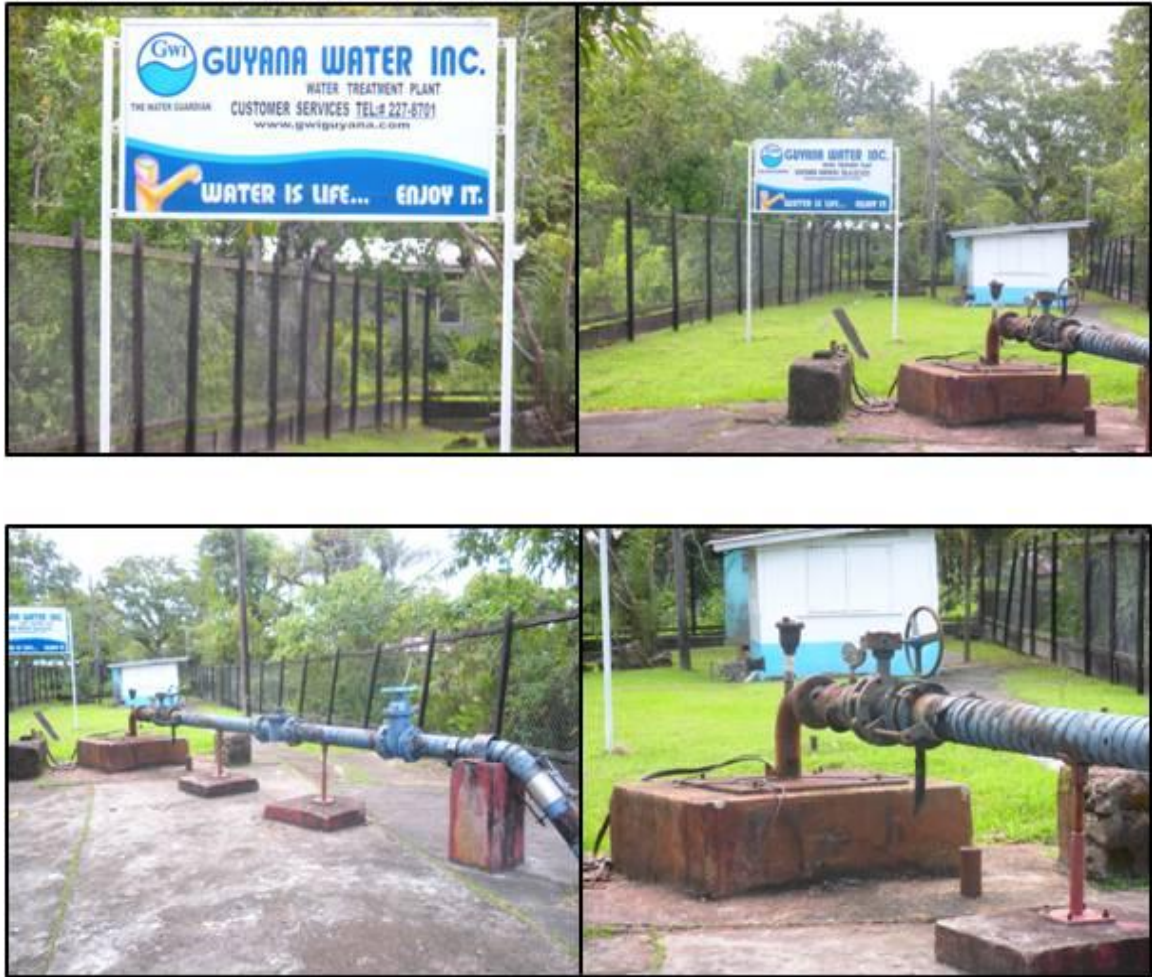
Figure D.8 Pictures from a Guyana Water Inc (GWI) treatment plant in Georgetown, Guyana.
