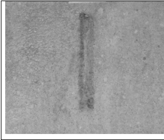
FIGURE 11(a) Digital Image of Longitudinal Concrete Crack a=5.4\text{mm} , d=2.5\text{mm}
