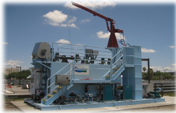
Figure 3.4 MBR Pilot System with Membrane A MBR Tank
