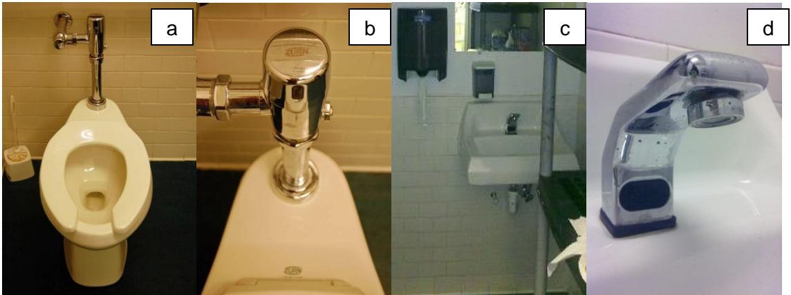
FIGURE 22: Photos of bathroom fixtures: (a) 1.28 gpf toilet, (b) detail view of sensor and manual button, (c) lavatory, and (d) detail view of faucet sensor.
