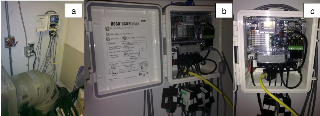
FIGURE 27: HOB0 data logger: (a) location in classroom closet, (b) sensor connections, and (c) detail inside view.
