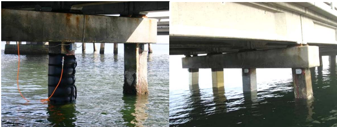
Figure 2.10 (a) Pressure bag on FRP wrapped pile; (b) Completed piles in bent.
