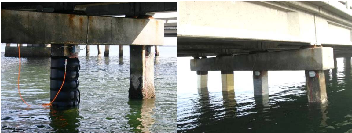
Figure 4.5 (a) Pressure bag on FRP wrapped pile. (b) Completed piles in bent.
