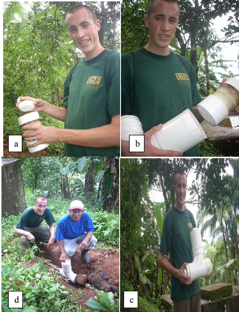
Figure 7: MINSA PVC Chlorinator in the Field. Clockwise from upper left: a) 3" diameter chlorine tablet being added to 3" PVC capsule; b) 3" PVC capsule inside 4" Tube; c) PVC chlorinator in the field; d) Chlorinator installed below ground surface upstream of water storage tank
