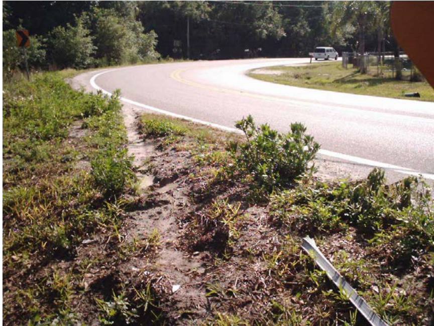
Figure 4.1: Recent run-off-road event in Site 1
