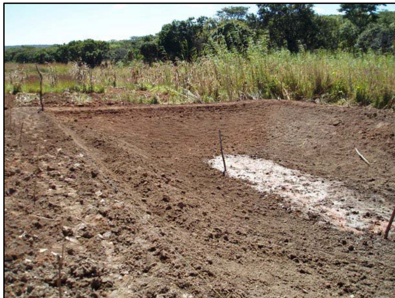
Figure L – Photo showing the completion of pond slope construction and leveling of dike walls
