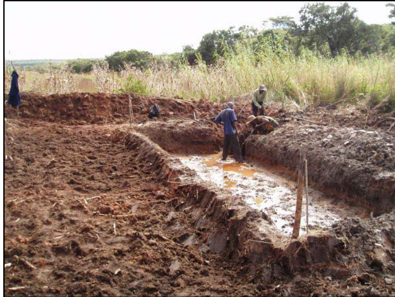
Figure K – Photo of pond construction after completion of the inner box
