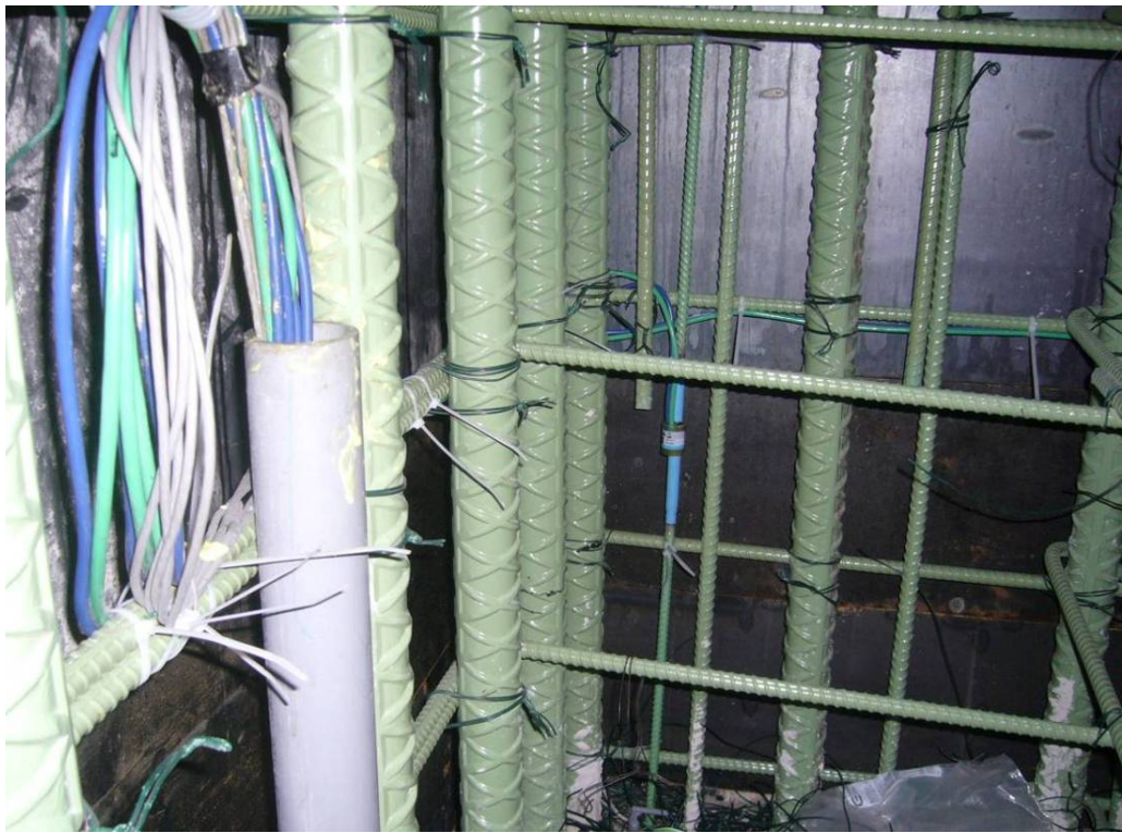
Figure 4-30: Gage Wires Exiting Through Conduit.
