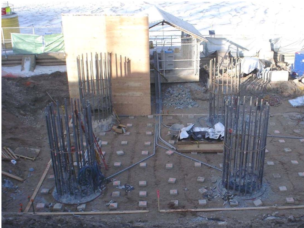
Figure 4-8: Conduits Running from Shafts to DAS Boxes.
