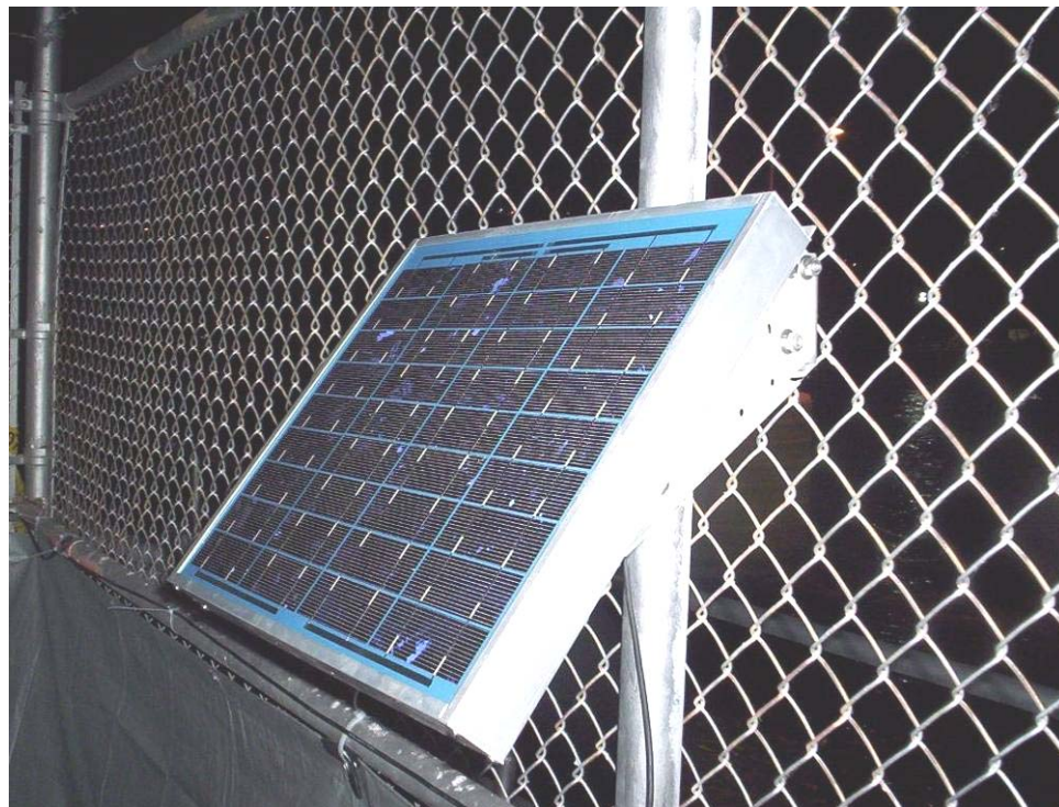
Figure 4-12: 35 Watt Solar Cell Panel for I-35W Bridge Monitoring System.
