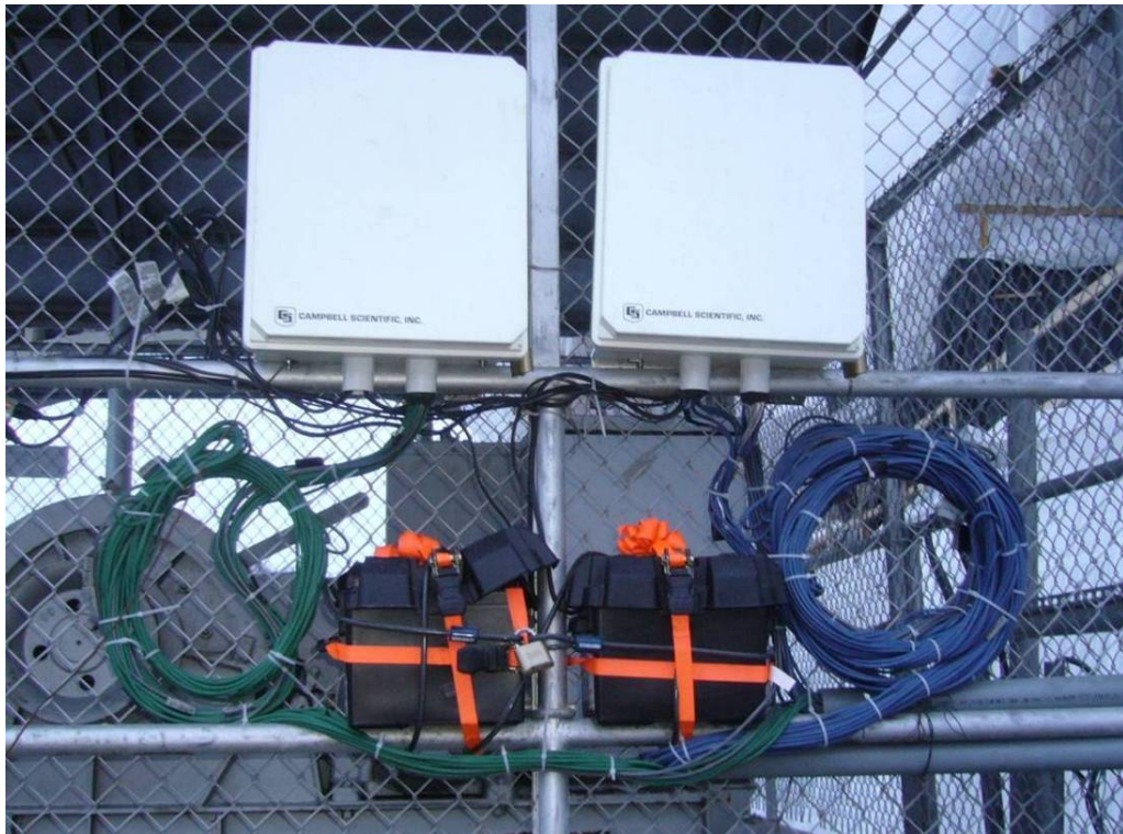
Figure 4-32: Construction Load Monitoring Systems. (VW – Blue, RT – Green)
