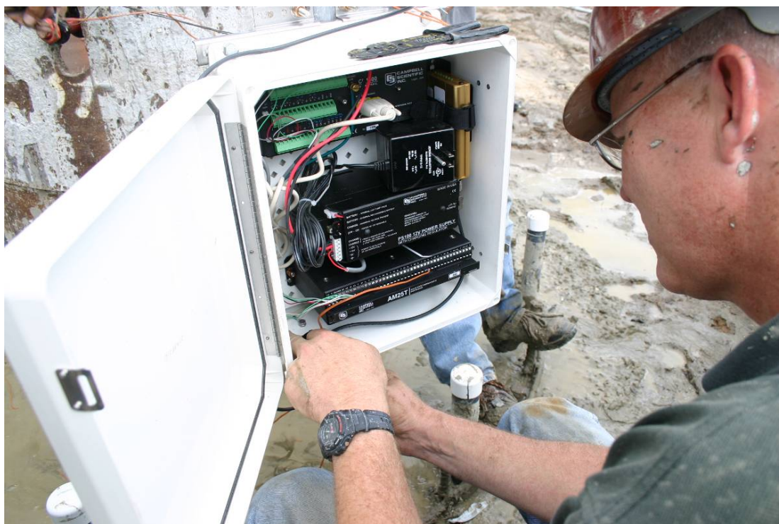
Figure 3-22: Thermocouple Wire Connection to AM25T to CR1000.
