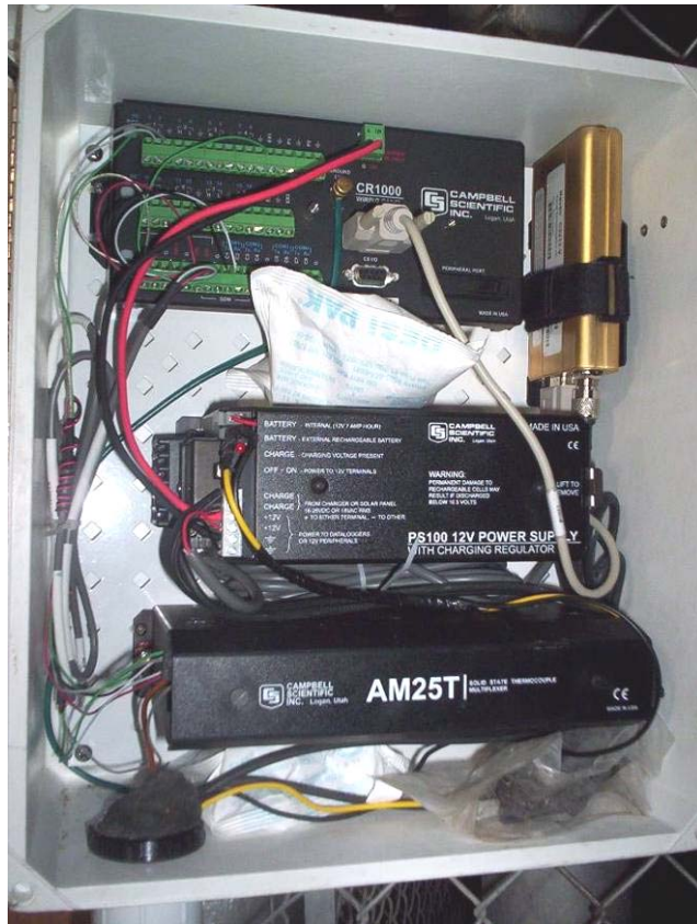
Figure 4-11: Thermal Monitoring DAS for I-35W Bridge Shafts.
