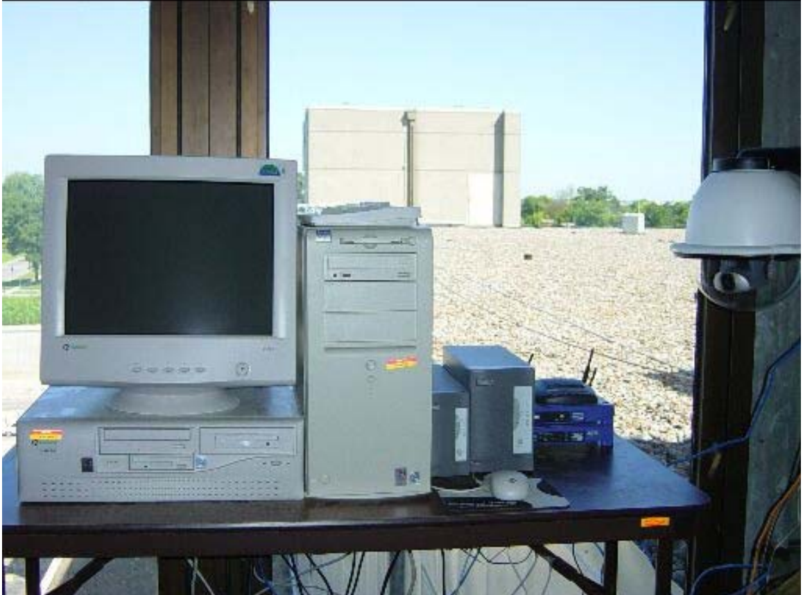
Figure 2-18: Dedicated Host Computer near Bridge Site. (Hemphill, 2004)
