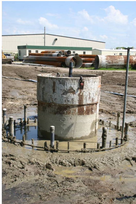
Figure 3-16: Final Voided Shaft at Ground Level.
