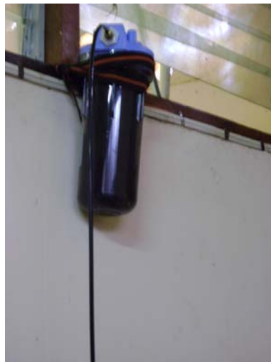
Figure 23 Filter used to treat rainwater for drinking purposes.
