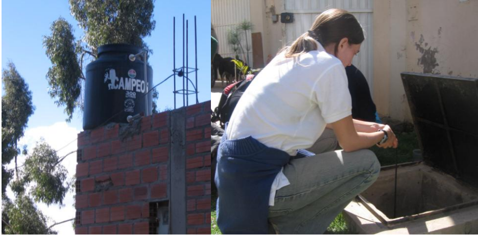
Figure 3: Elevated storage tank and cistern photos. a) Elevated water storage tank located on the roof of a home; b) Underground cistern located next to home near street.
