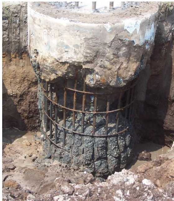
Figure 1.1: Drilled Shaft with Concrete Void
