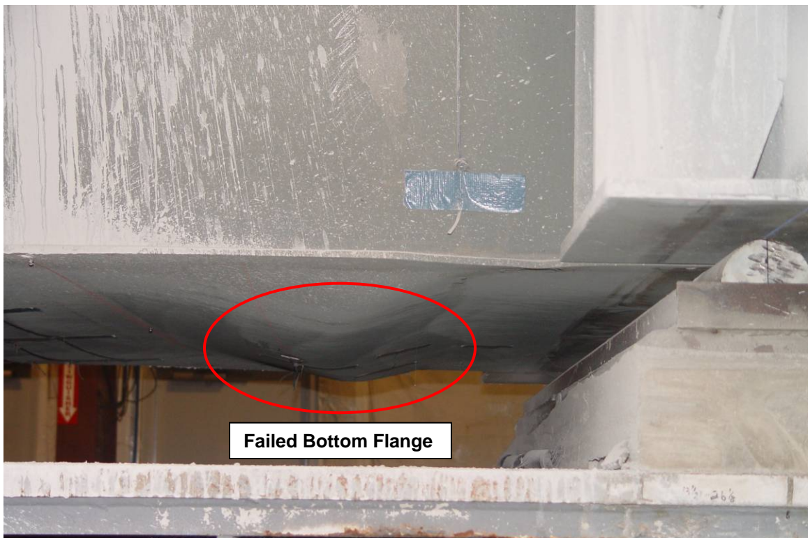
Figure 3.16 Failed Bottom Flange on Hold Down Side
