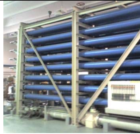
Blue Pressure Vessels on Skid 4
