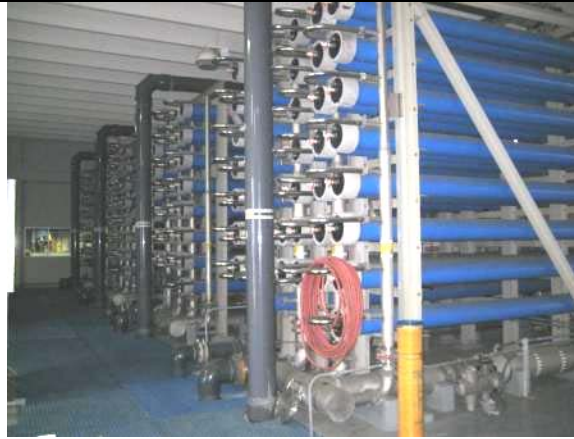
Four Skids at DWTP
