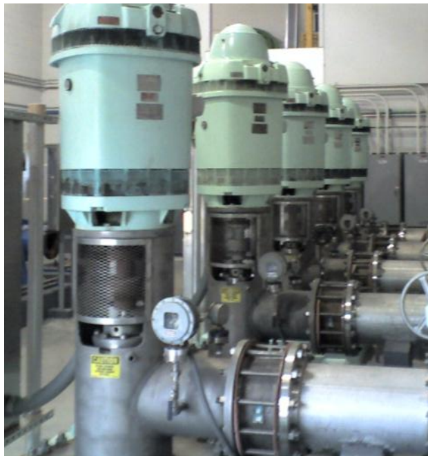
Feed Water Pumps Just After Anti-scalant Injection
