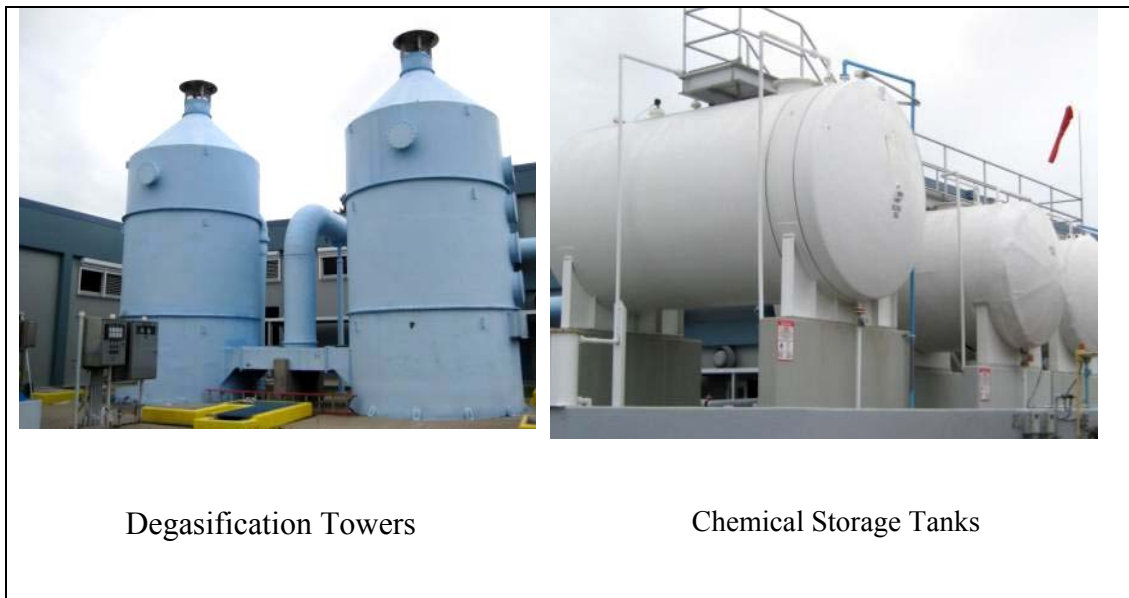
Figure 4: Pictures of Various Post Treatment Systems
