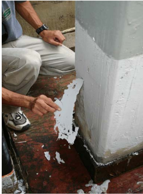
Figure 3.9 Peeling Off Unbonded Resin
