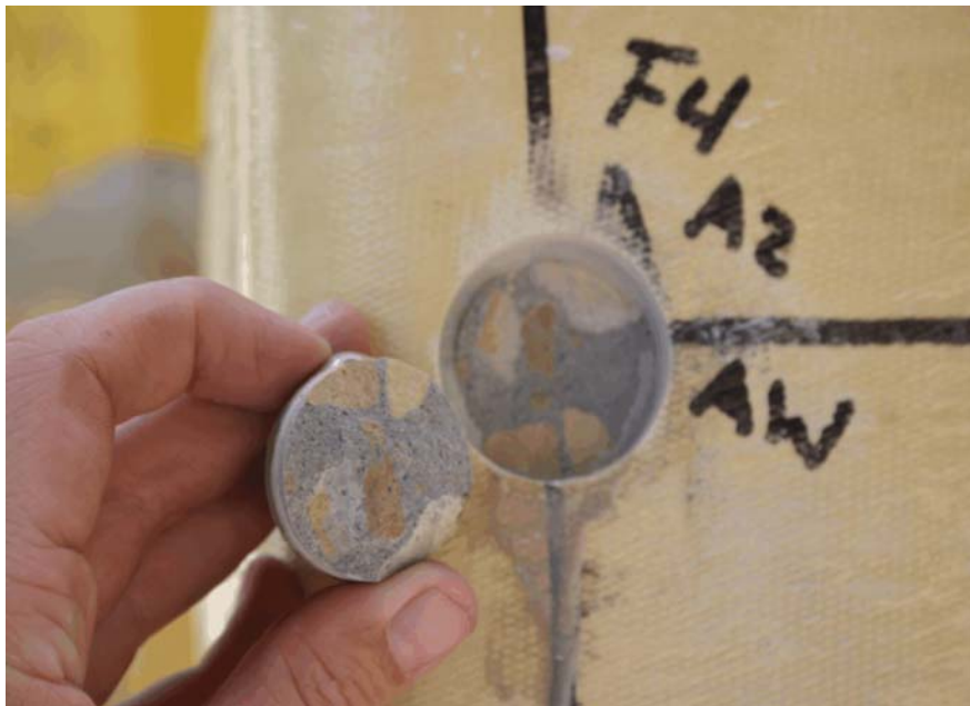
Figure 4.6 Full Concrete Failure of Pull-off Test
