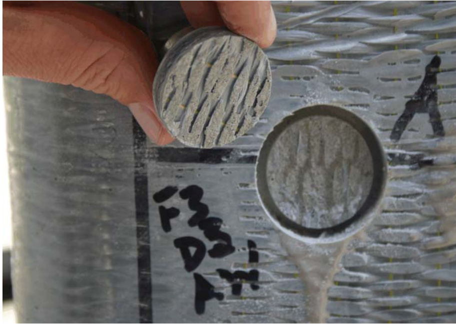
Figure 4.5 FRP Failure of Pull-off Test
