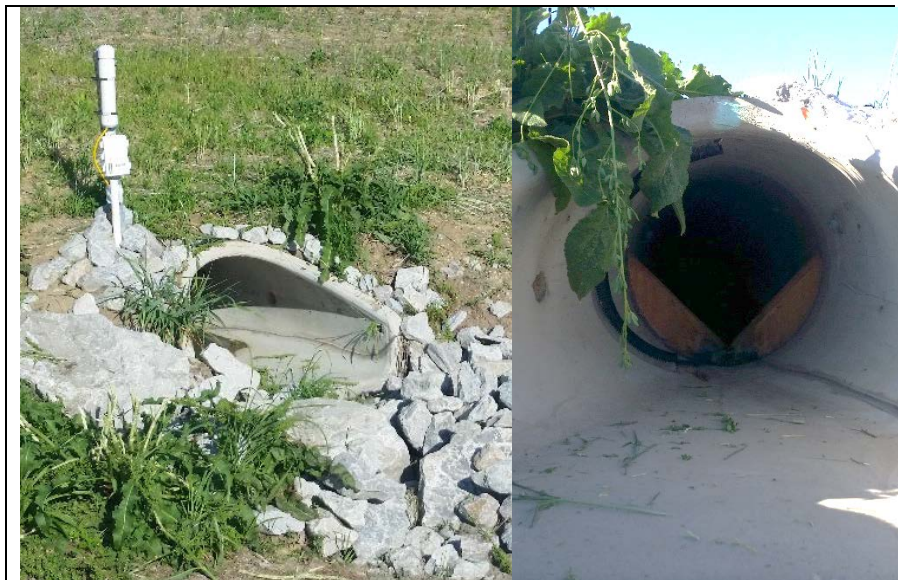
Figure 3: Internal and external setup of cell inlet apron instrumentation
