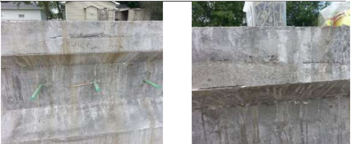
Figure 5-13 Cold Joints Appeared on Second Girder
