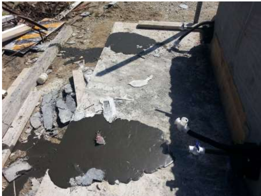
Figure 5-24 Grout Appeared Darker than Surrounding Concrete
