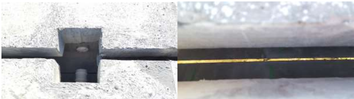
Figure 5-30 Gaps Created at Each Joint
