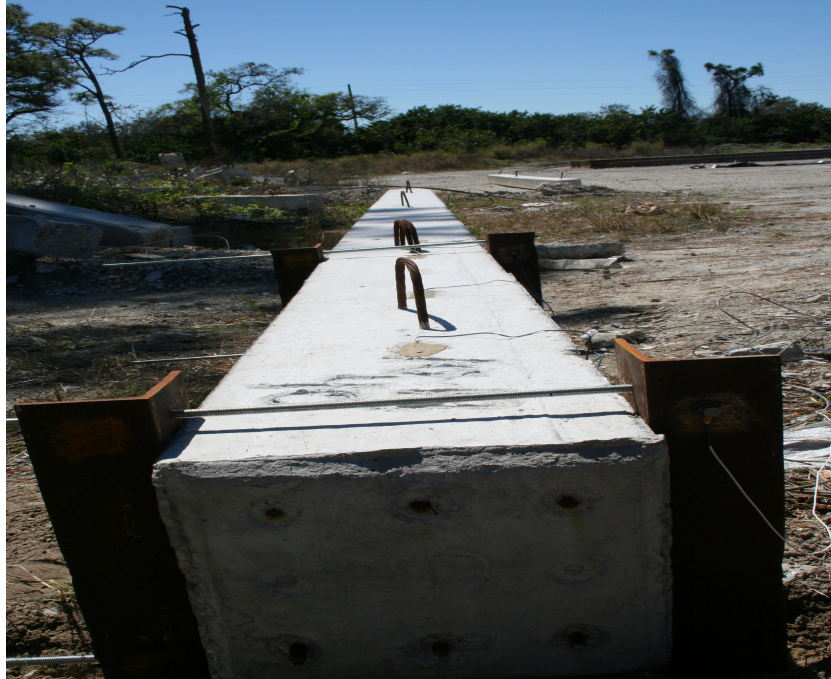
Figure 3.5: Pre-stressed Concrete Piling 12”x 12”x 40’
