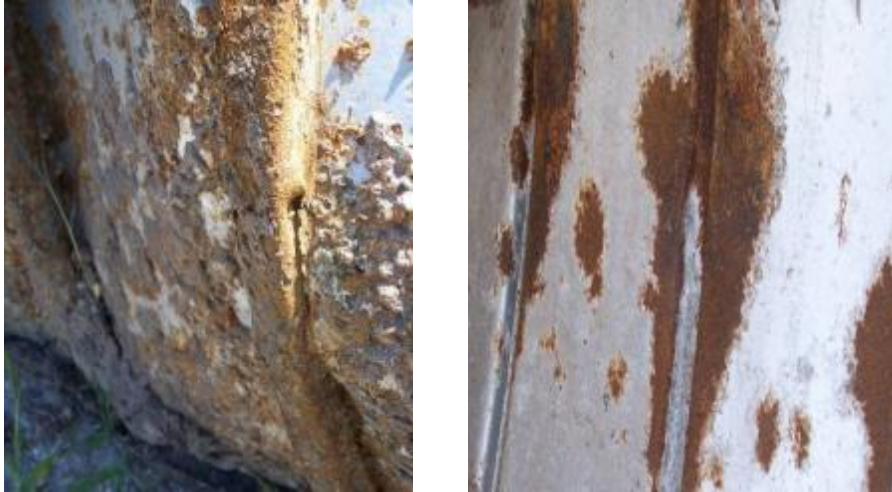
Figure 1-4. Corroded Pipe from the Curlew Rd. Site, Pinellas County, Fla. (2007) [Photograph by the Author].
