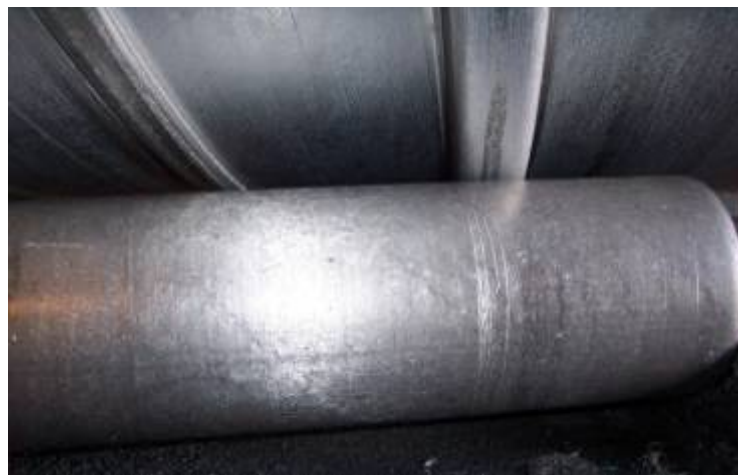
Figure 1-3. Minor Scratches During Fabrication Spiral Rib Pipe. [Photograph by the Author].
