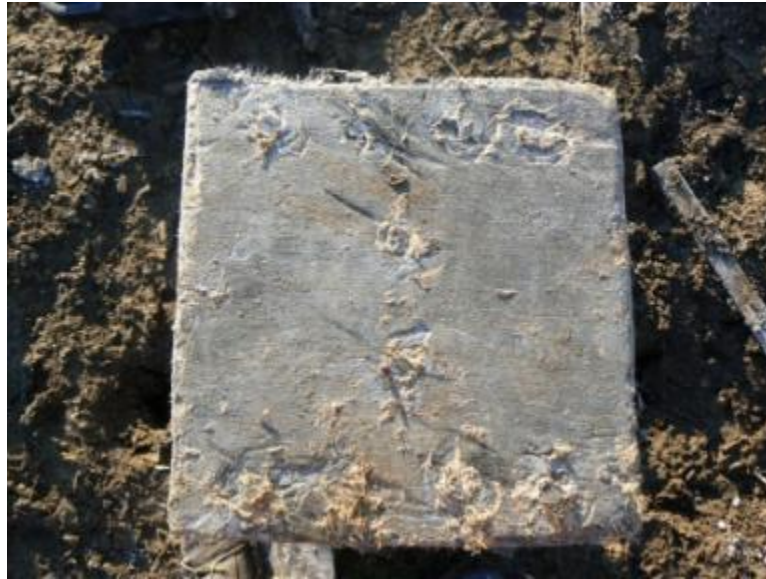
Figure 5.12. Condition of pile head at the end of driving pile P2
