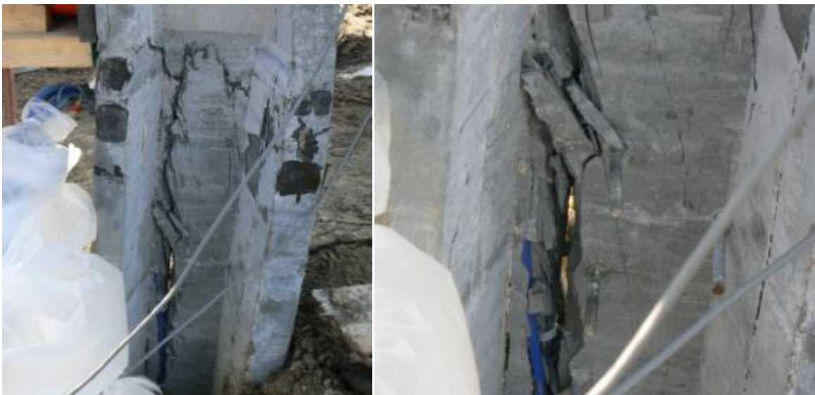
Figure 5.44. Views of the shear cracking on the east side of the web of UHPC pile P1
