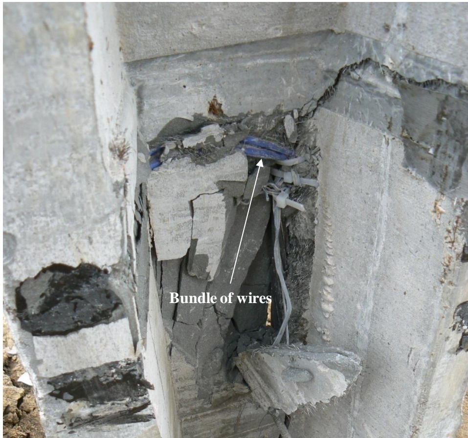
Figure 5.49. Shear failure region of UHPC pile P1 after the lateral load test with some cracked UHPC pieces removed
