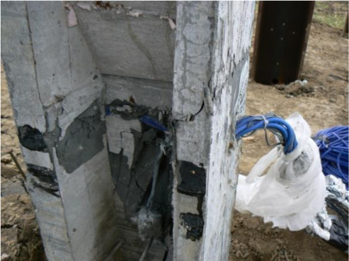
Figure 5.48. Bundle of instrumentation wires passing through the web and out of the flange of UHPC pile P1
