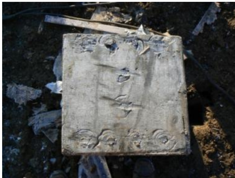
Figure 5.13. Condition of pile head at the end of driving pile P1
