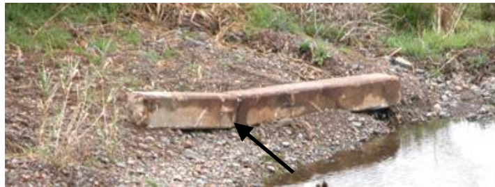
Figure 1.1. Precast, prestressed concrete pile cracked during driving (RTA NSW 2005)
