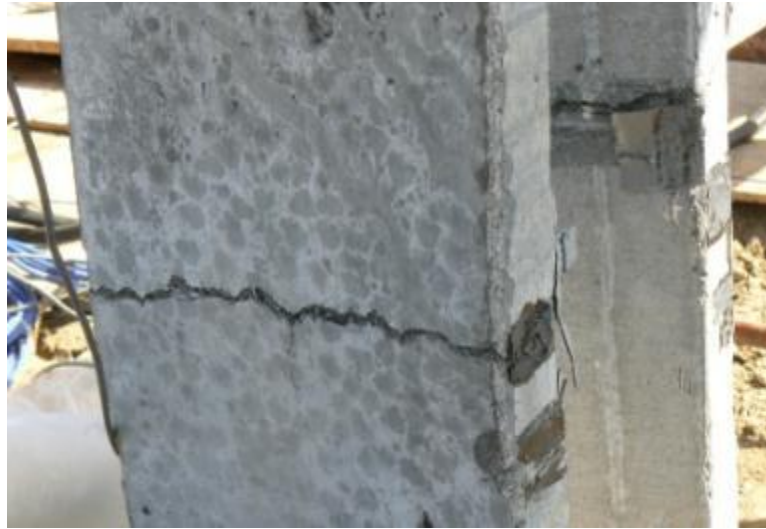
Figure 5.45. Cracking of back flange of UHPC pile P1
