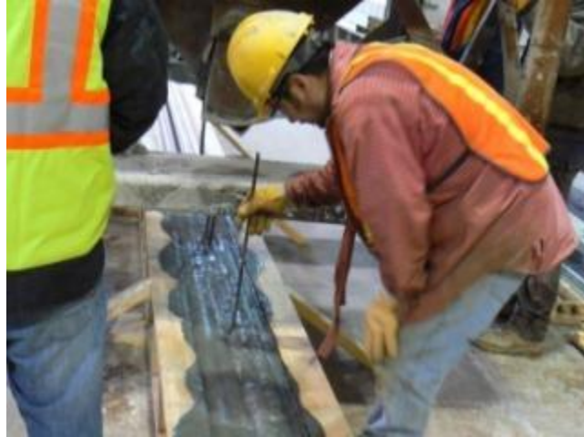
Figure 4.24. “Rodding” through the web of UHPC to eliminate formation of possible air pockets
