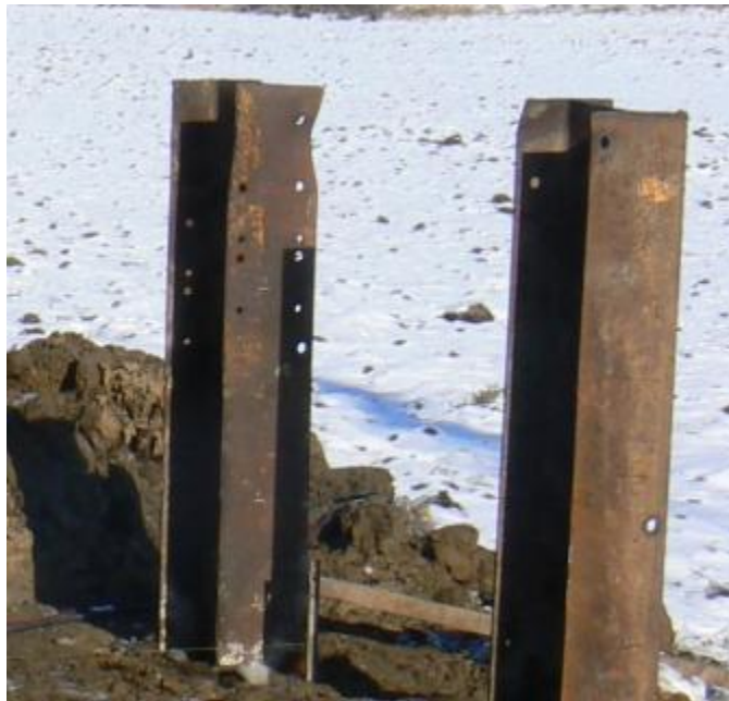
Figure 5.8. Local buckling and bending damage to two steel anchor piles due to driving
