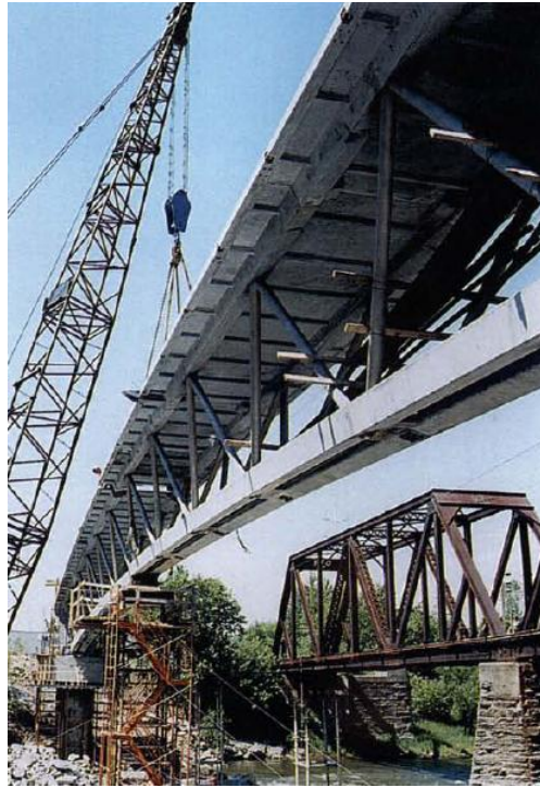
Figure 2.38. Placement of the second half segment of the Sherbrooke bridge on the falsework bent (Blais and Couture 1999)
