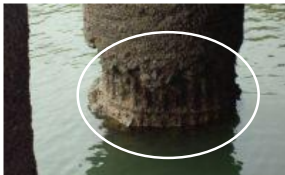
Figure 1.4. Prestressed concrete marine pile with spalling and reinforcement corrosion in a marine environment (Port Strategy 2007)
