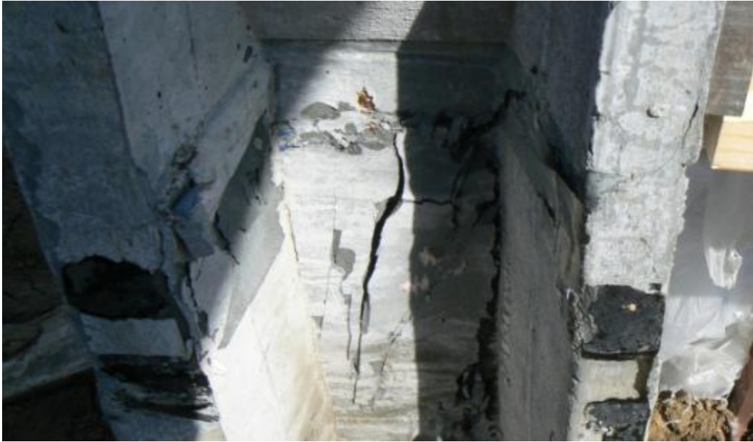
Figure 5.43. Initial shear cracking in web of UHPC pile P1 at a lateral load of 22.8 kip (101.3 kN)
