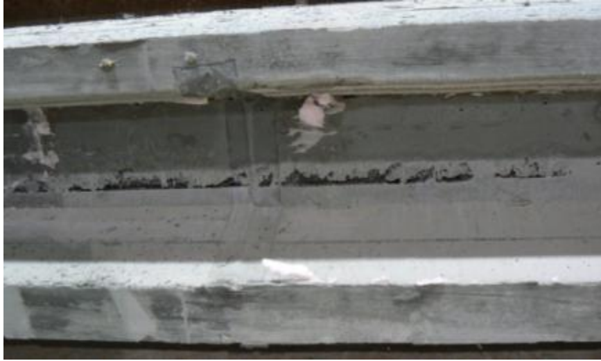
Figure 4.21. Minor pocketing observed in the web of UHPC pile P1
