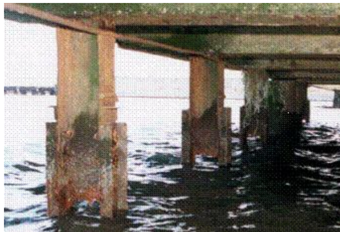
Figure 1.8. Corroded steel piles with loss of section in a marine environment (Juran and Komornik 2006)
