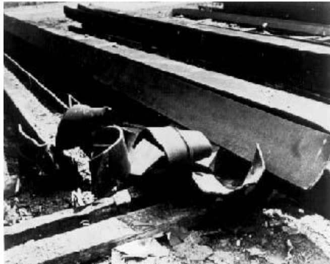
Figure 1.5. Steel piles heavily damaged due to hard driving (DiMillio 1998)
