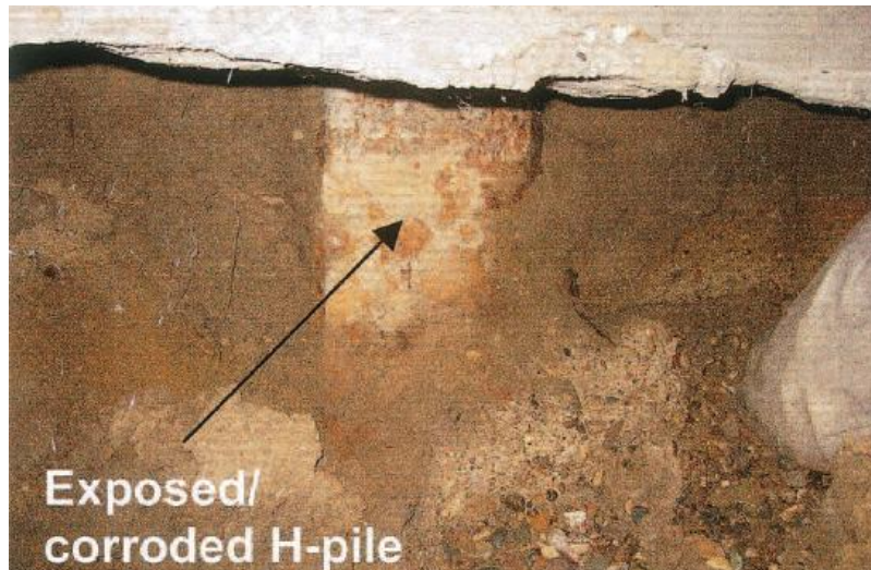
Figure 1.9. Corroded H-pile supporting integral abutment (White et al. 2007)
