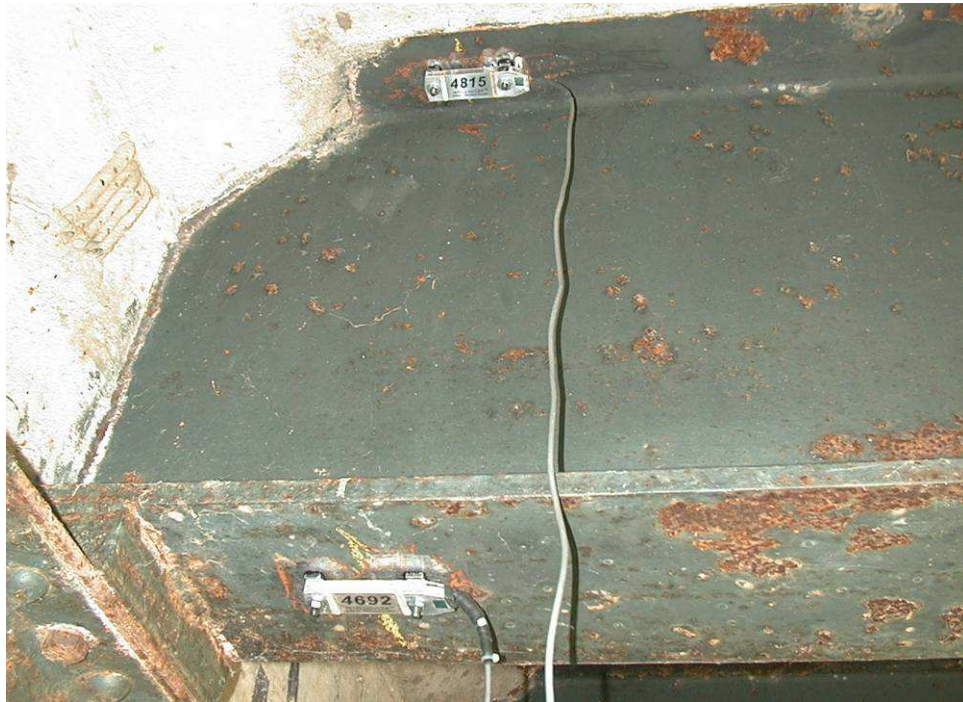
Figure 4.8. Instrumentation Near Abutment of MCB.
