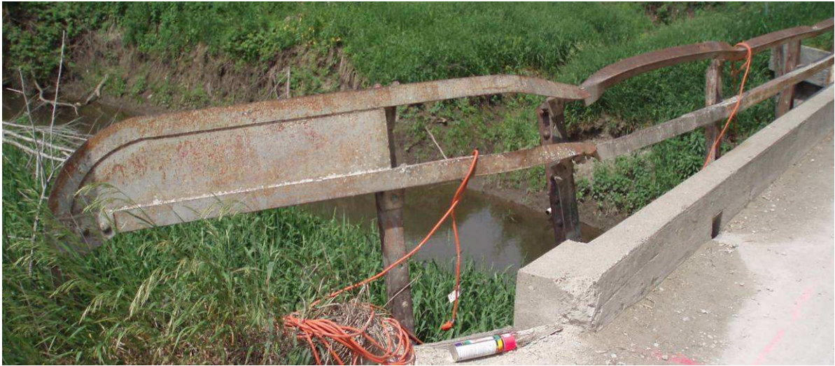
Figure 7.3. KCB2 Railing Damage.
