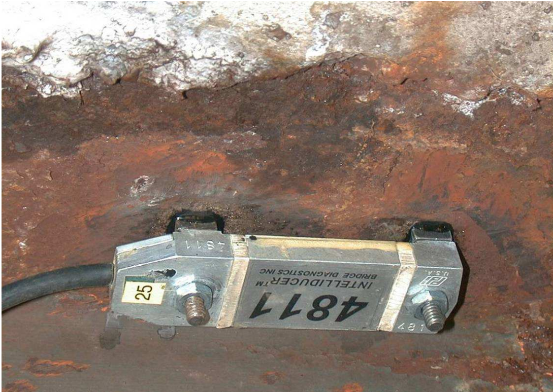
Figure 4.11. MCB Removal of Excess Corrosion for Transducer Application
