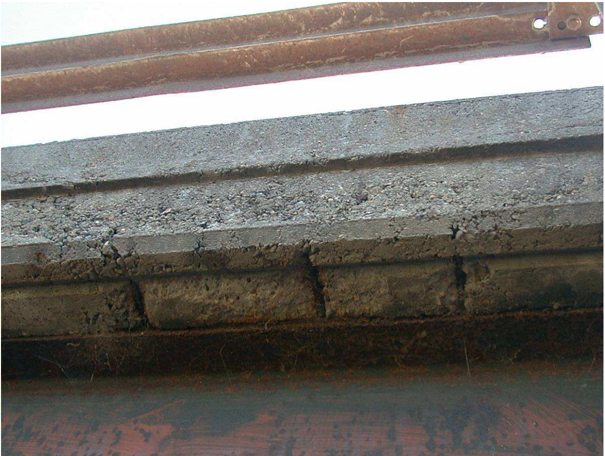
Figure 5.2. KCB1 Poor Concrete Consolidation.
