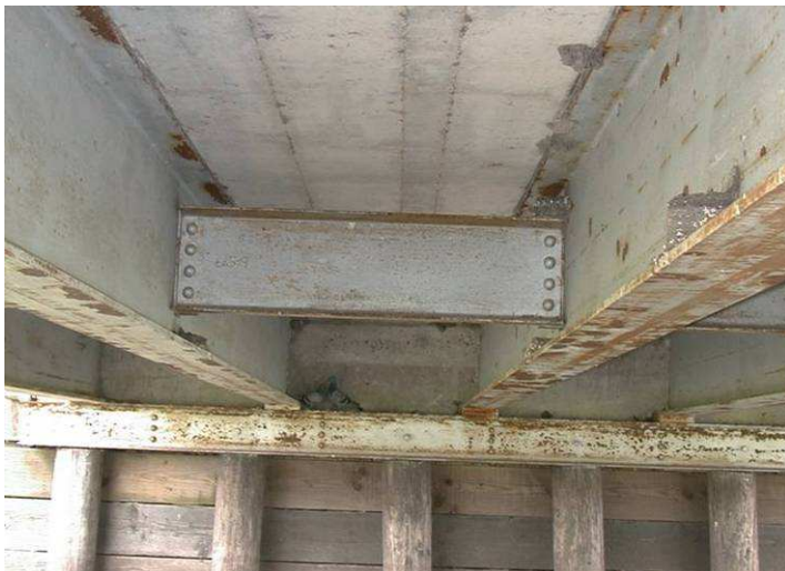
(a) Minor rust on girders
