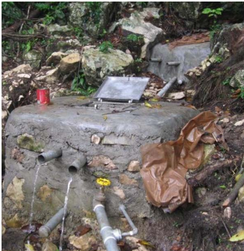
Figure 16: Protected spring water is collected through a springbox and reservoir constructed using metal pipes, cement, and bricks (Photo: C. Prouty)
