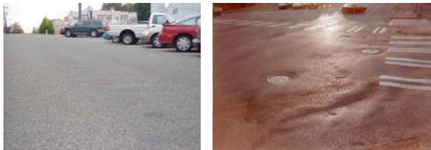
Figure 2.3 Corrugation (left) and Shoving (right) in the Asphalt Pavement Surface (8).
