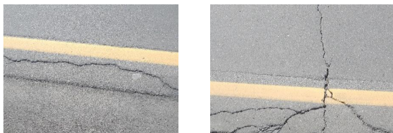
Figure 5.17 Medium Severity Edge Cracks from Minnesota Test Sections.
