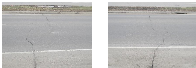
Figure 5.16 Medium Severity Transverse Cracks from Minnesota Test Sections.
