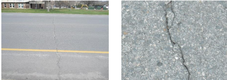
Figure 5.8 Medium Severity Joint Reflection Cracks from Iowa Test Sections.
