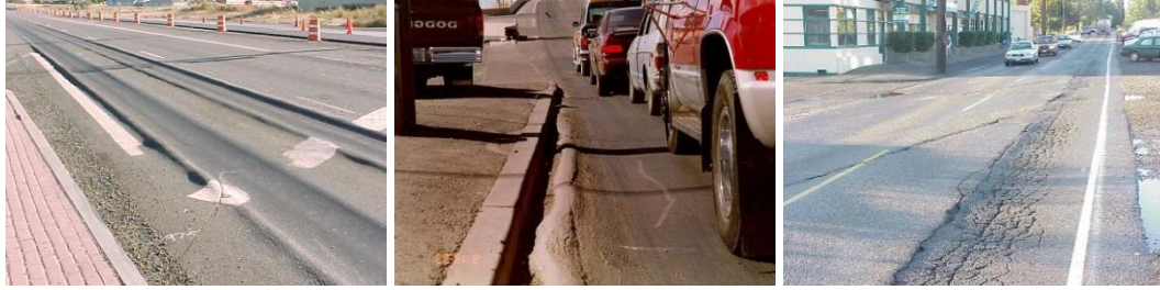
Figure 2.1 Sever Mix Rutting (left), Mix Rutting (middle), and Rutting in the Wheel Path (right) (8).
