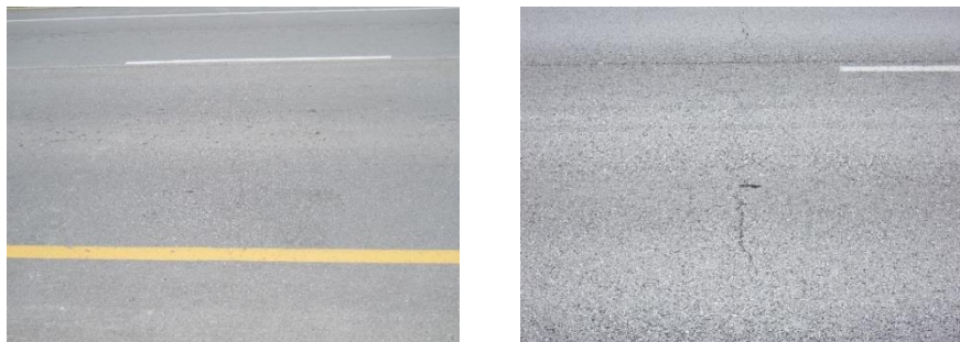
Figure 5.10 Low Severity Slippage Cracks from Iowa Test Sections.
