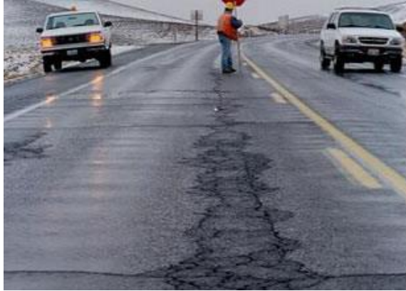
Figure 2.18 Fatigue Cracking Caused by Stripping (18).
