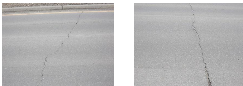
Figure 5.15 Medium (left) and High (right) Severity Joint Reflection Cracks from Minnesota Test Sections.
