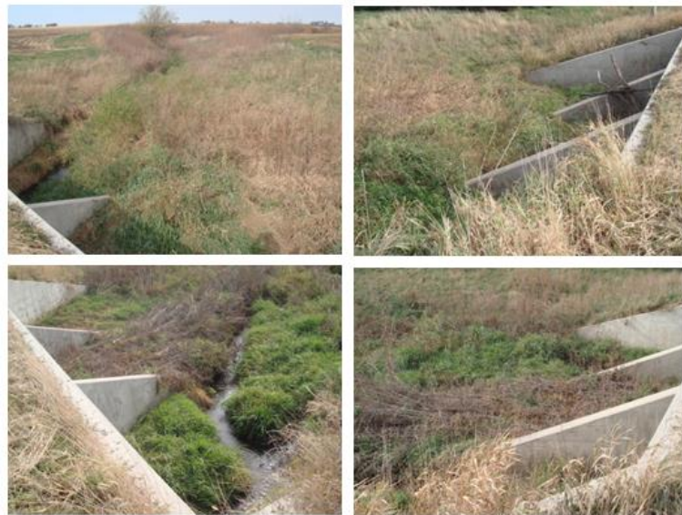
Figure 1.11 Culvert siltation observed through previous studies (M Muste et al., 2009): a) 3-box culvert located on the Old Mill Creek in Solon; b) 3-box culvert located on the North Branch Volga River
