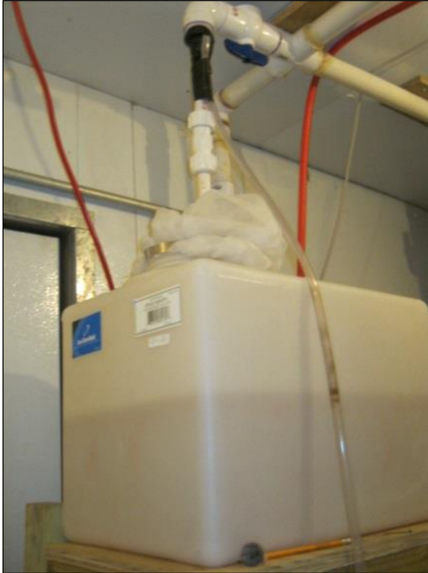
Figure A3. An image of the influent piping system and dose tank.
