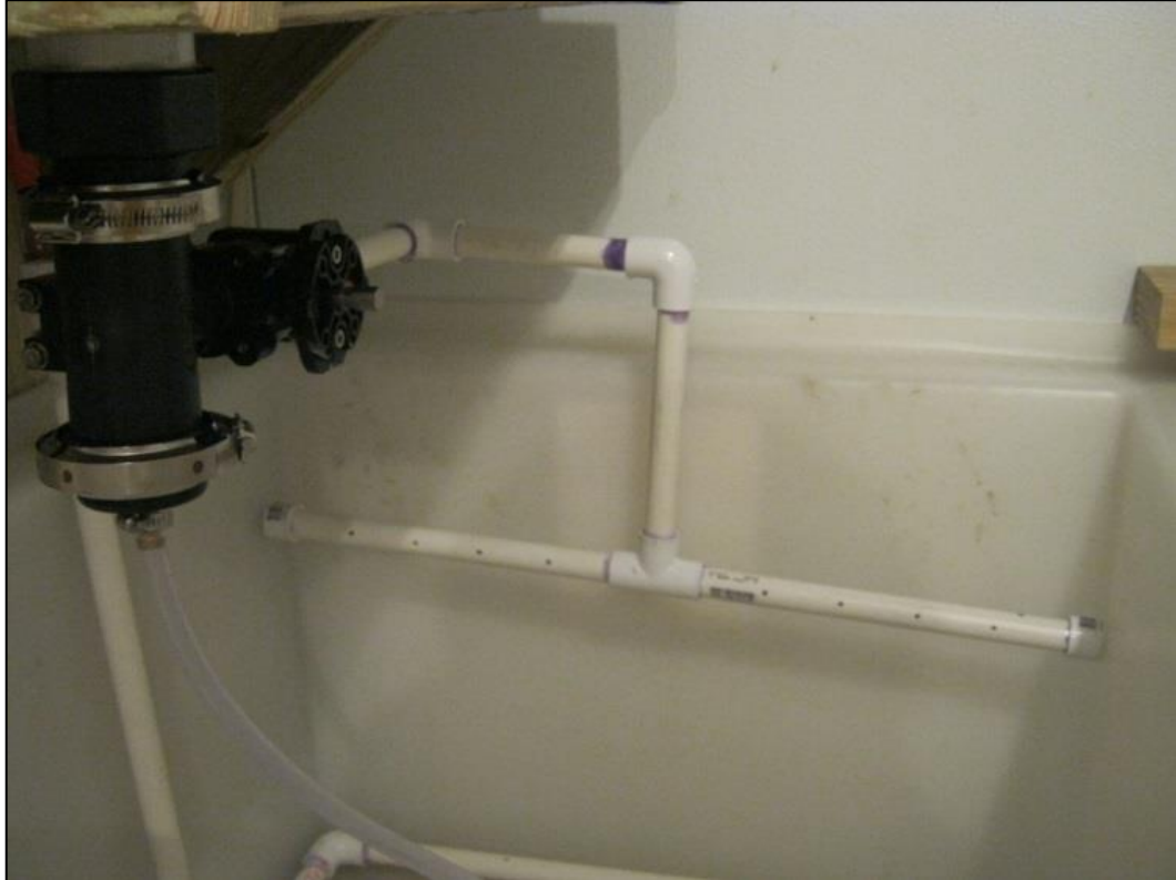
Figure A5. An image of the influent manifold (PVC pipe) before the addition of pea gravel.
