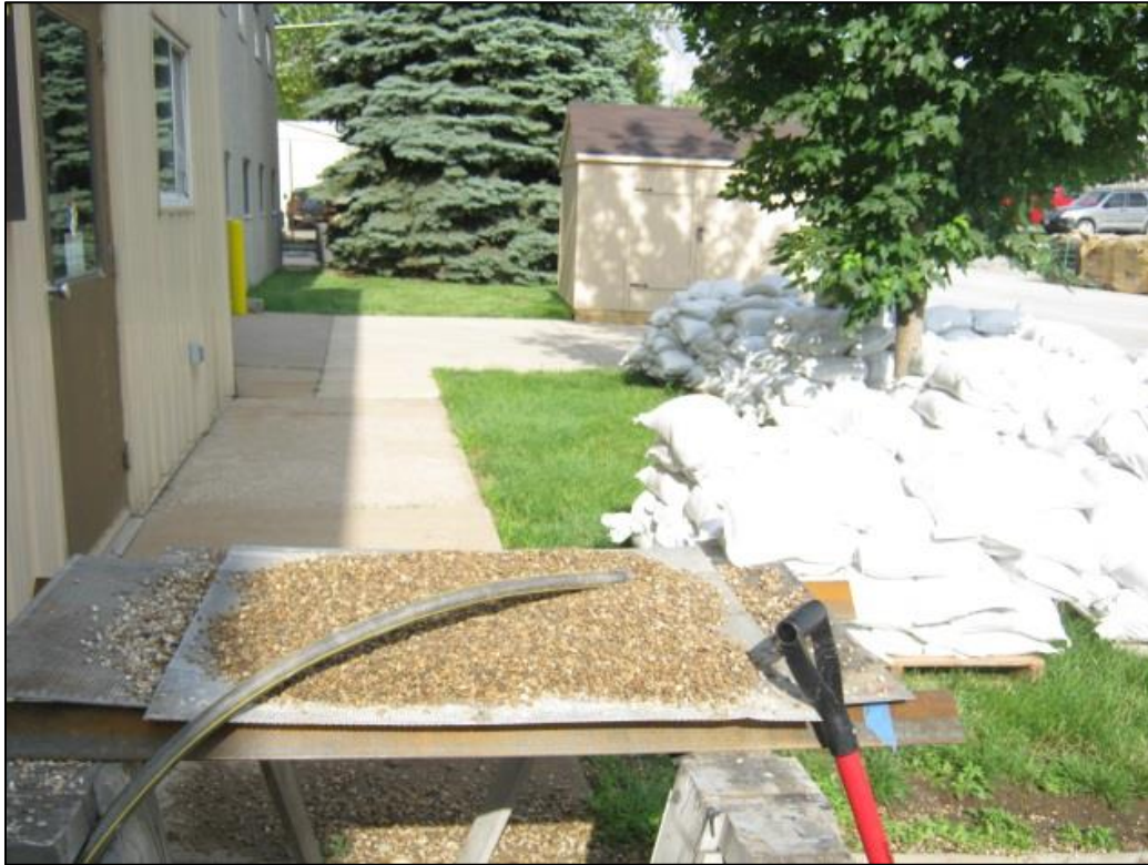
Figure A11. An image of the setup used to wash the pea gravel.
