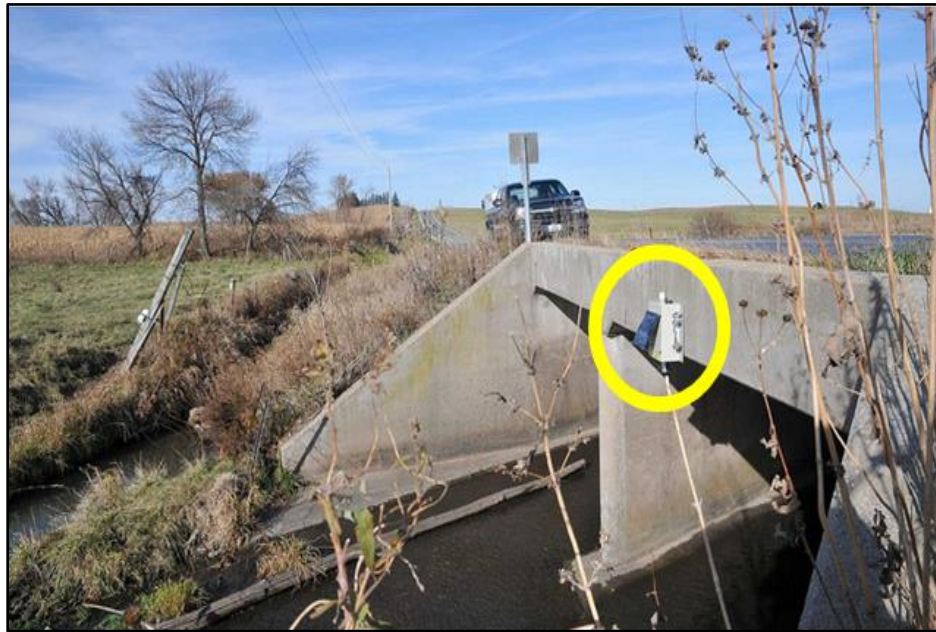
Figure 1.2: USBS installed on a Bridge crossing at Buffalo Creek, Johnson County. (Photo Courtesy of Iowa Flood Center)
