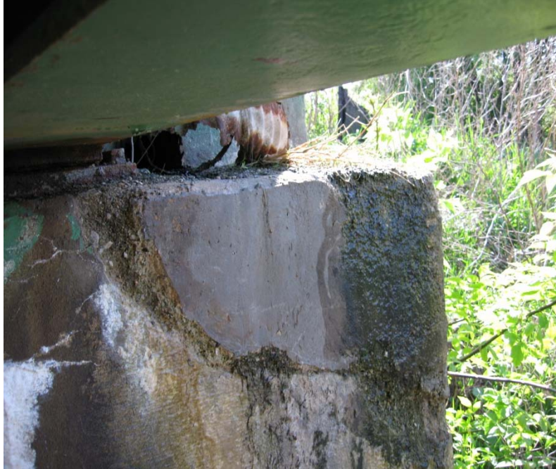
Figure 4.45 Large diagonal crack in the northeast abutment wall beneath beam 4
