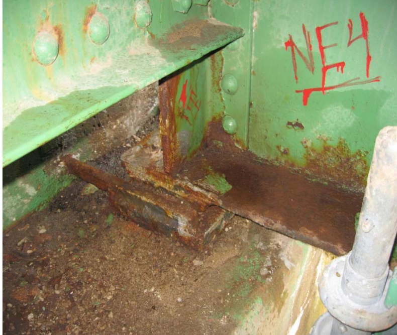
Figure 4.48 Forced vibration response measurement of northeast end and boundary condition of beam 4 with noticeable deterioration of the bottom flange
