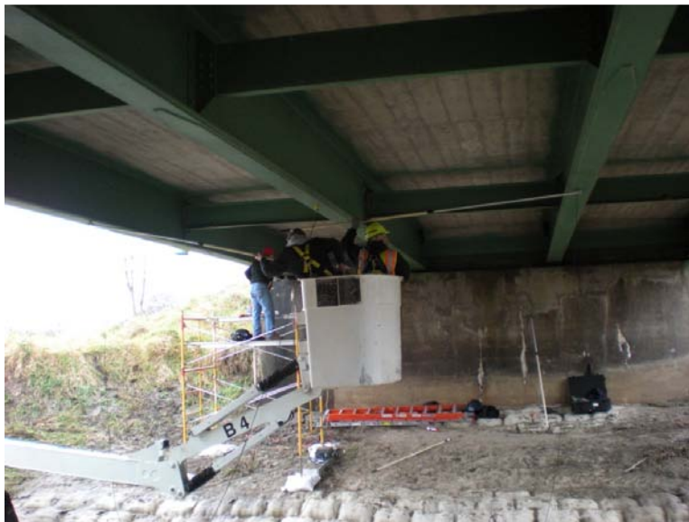
Figure 4.7 Snooper truck and long poles used to access the bottom flange of each beam
