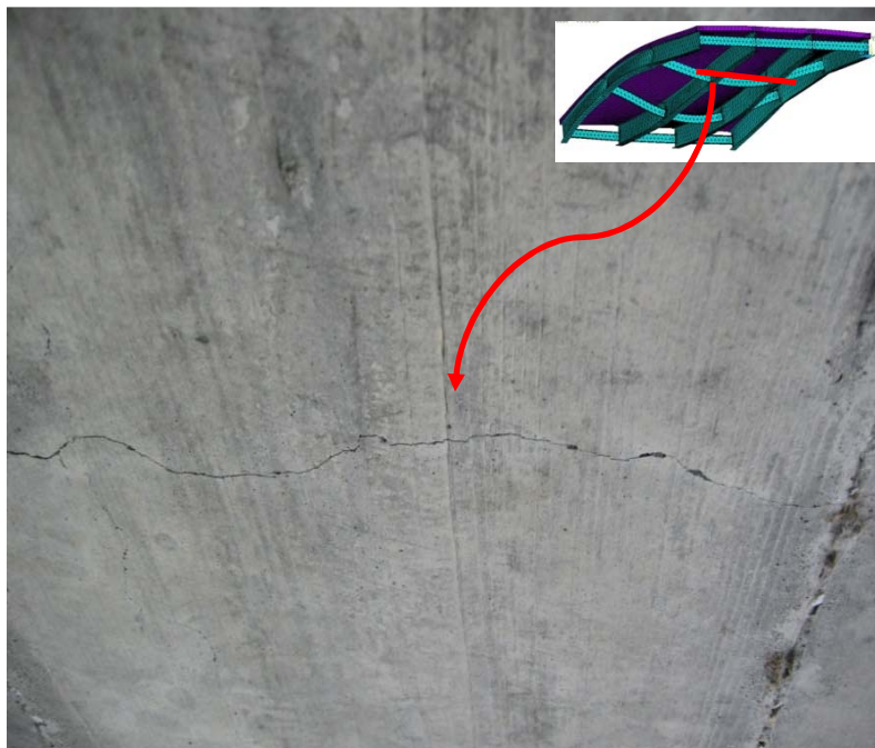
Figure 4.41 Lateral surface crack in concrete deck near midspan of bridge
