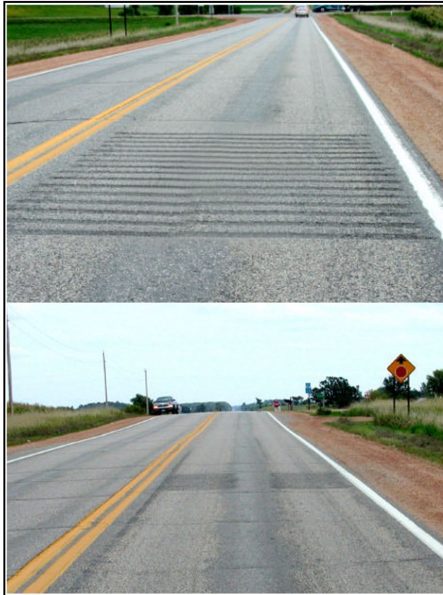
FIGURE 30. In-lane intersection approach rumble strips (47)
