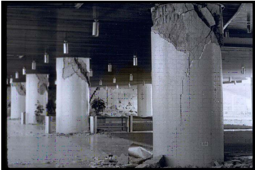
Figure 1-2: Damage to the 2 nd Story Columns of the Macuto Sheraton due to the Caracas Earthquake [2]
