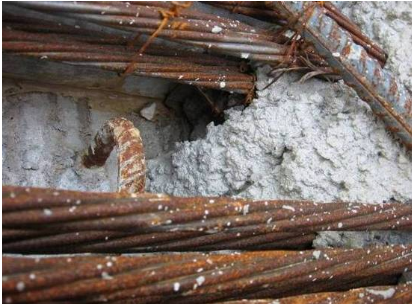
b) concrete flowing between post-tensioning strands
