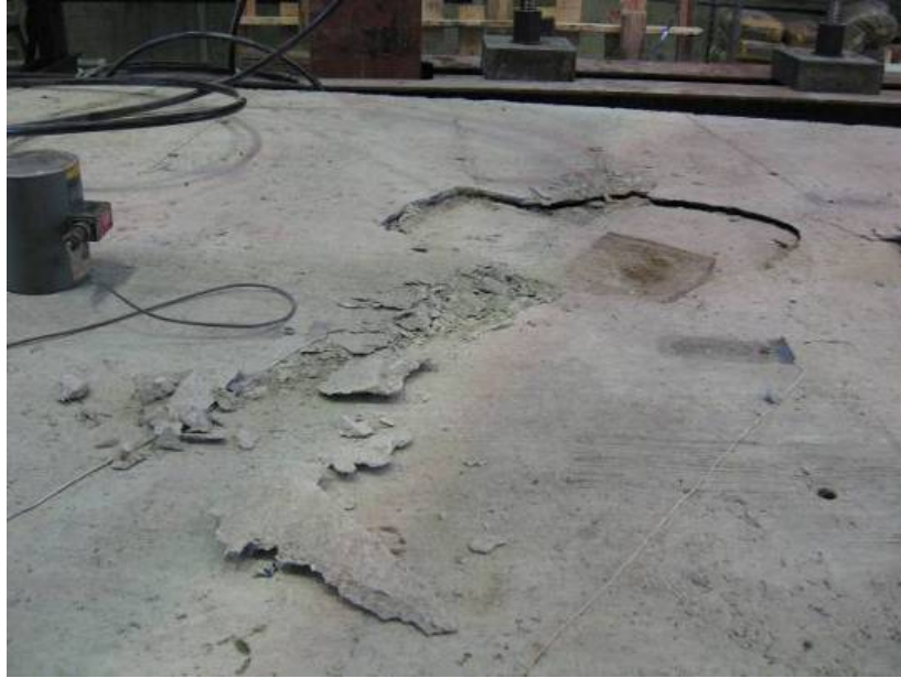
Figure 3.25. Punching shear and flexure failure due to tandem wheel footprint.
