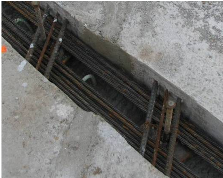
Figure 2.17. Photograph of longitudinal post-tensioning channel prior to casting concrete in the field.
