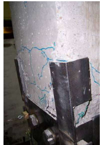
b.) Upper column segment damage
