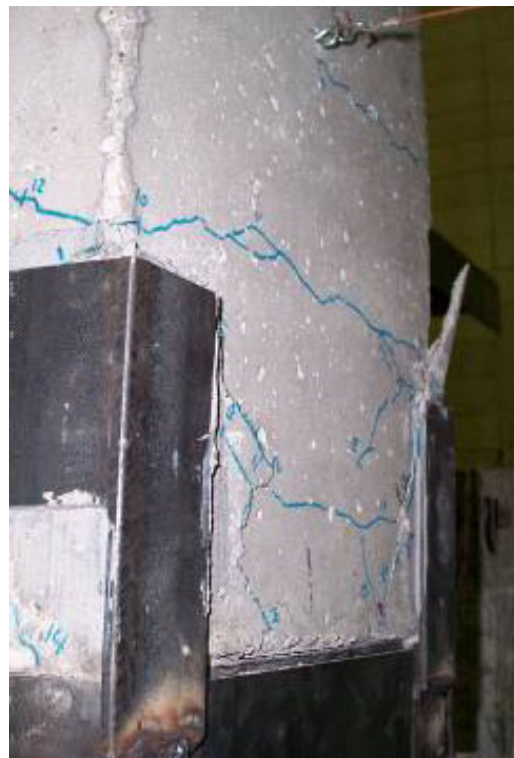
Figure 114. Photograph of Column 4 – Cycle 19b west face of upper column segment.
