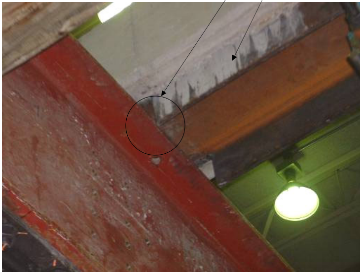
a.) Frame impingement with underside of load beam
