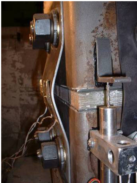
a.) East fuse plate buckling
