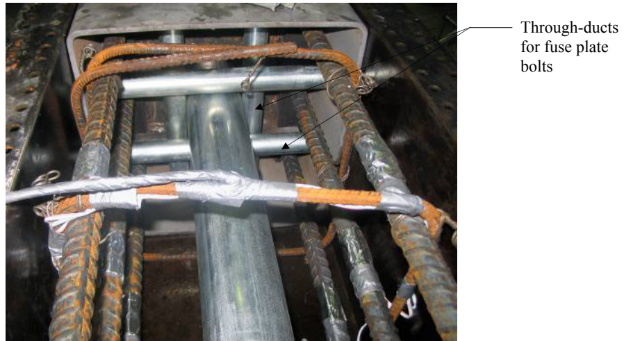
Figure 55. Photograph of Column 5, 12 ft. segment collared end.
