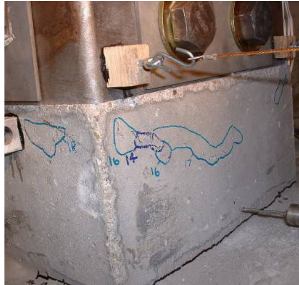
b.) Northwest corner compression damage
