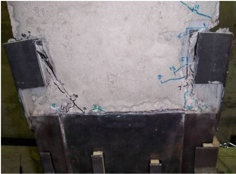
c.) North face damage and retrofit angle failure
