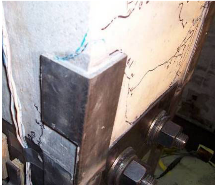
b.) Incipient cracking at southeast retrofit angle
