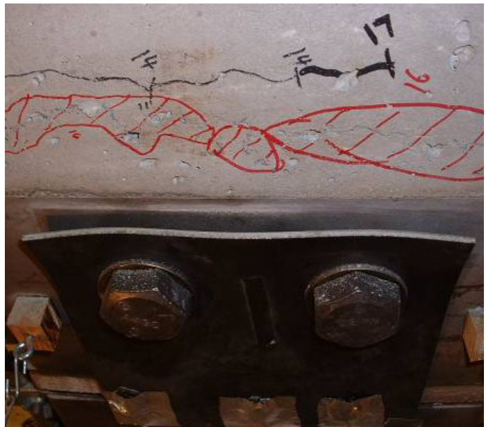
b.) Bolt bearing on west fuse plate causing plate curling
