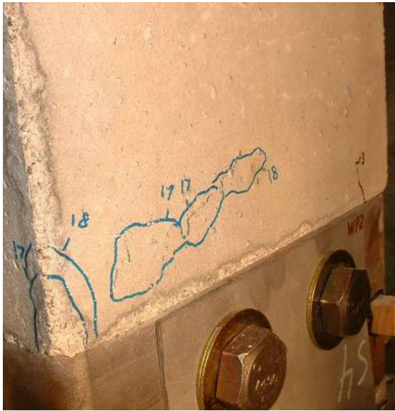
a.) Upper west column segment compression damage
