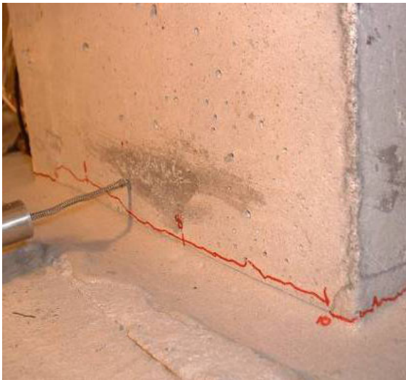
a.) East face initial cracking
