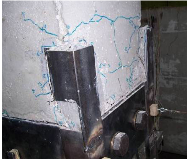
b.) Upper segment damage and retrofit failure
