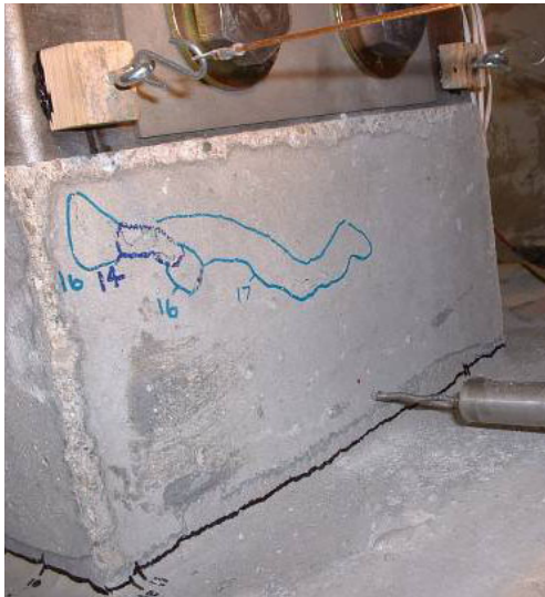
a.) West face initial compression damage
