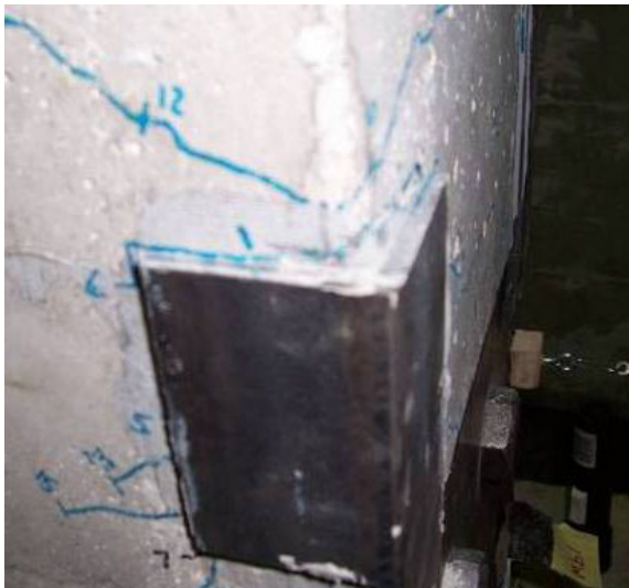
a.) Cracks forming around southeast retrofit angle
