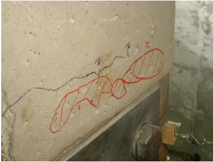
a.) Upper segment compression damage
