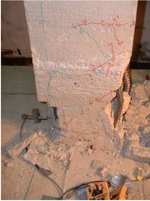
a.) South view of damage
