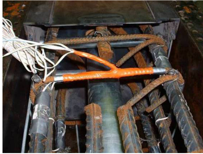
Figure 47. Photograph of Column 4 collar region congestion.
