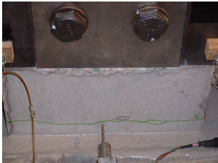
b.) West base initial cracking
