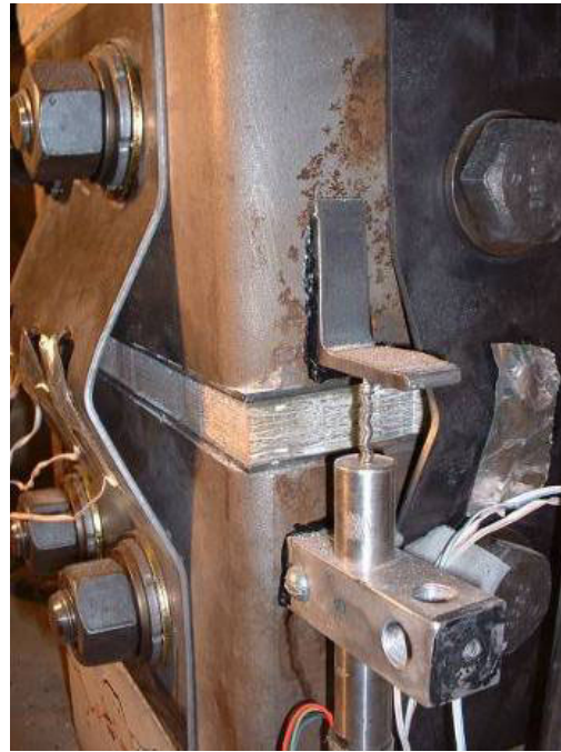
b.) East fuse plate buckling
