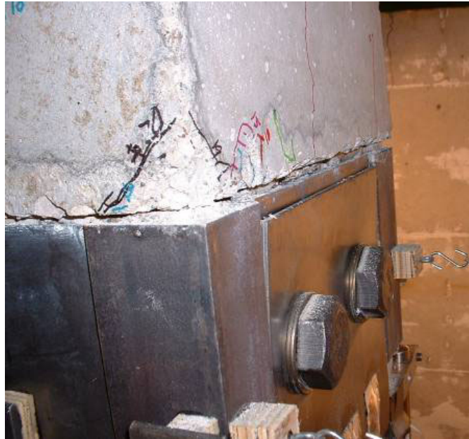
b.) West collar/column interface final crack width
