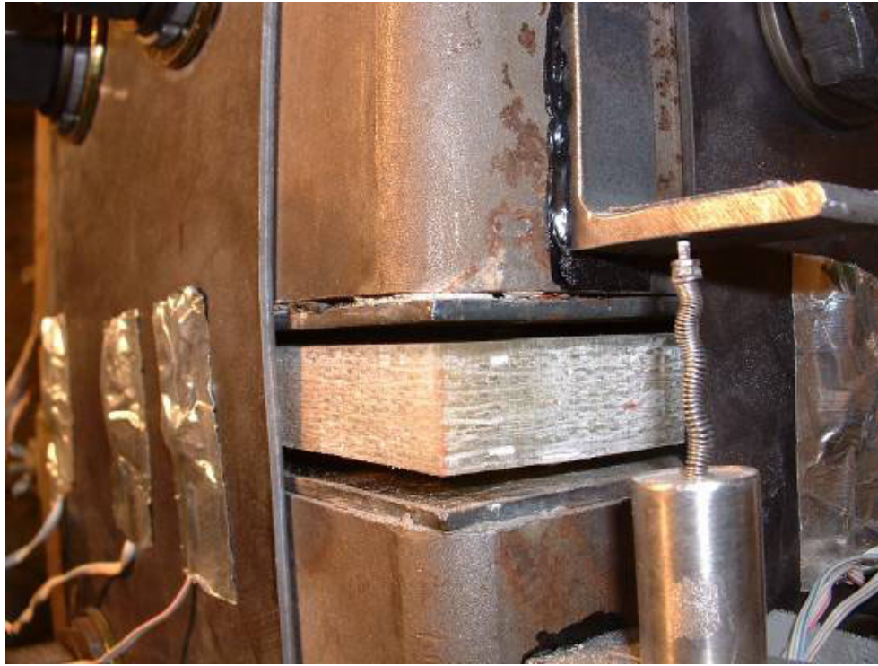
a.) Northeast corner joint opening
