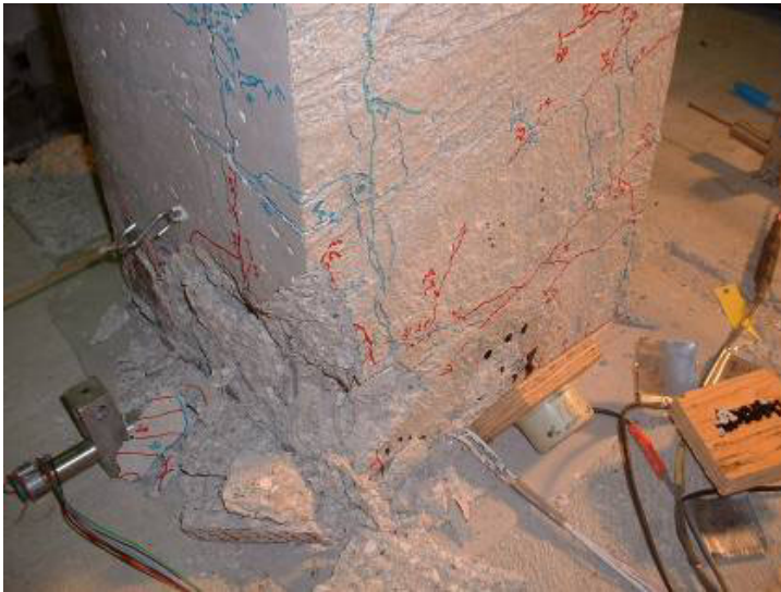
a.) Severe spalling of southwest corner
