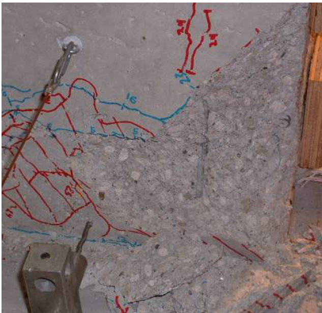
a.) Southwest corner damage
