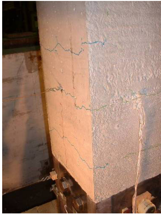
b.) Southwest corner crack progression
