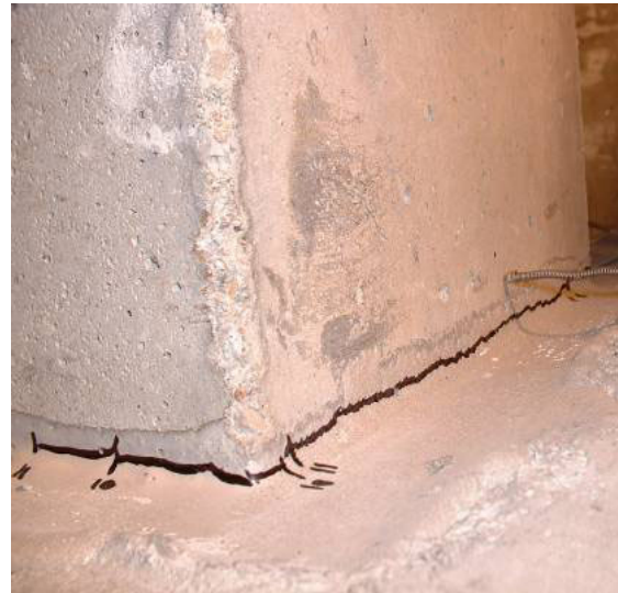
b.) West face initial cracking
