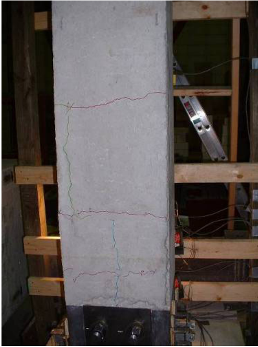
a.) East face crack progression
