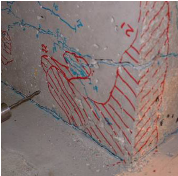
a.) Southwest corner compression damage
