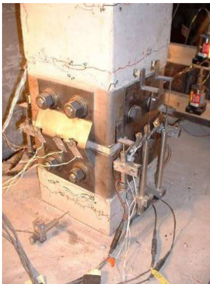
a.) Residual fuse plate buckling
