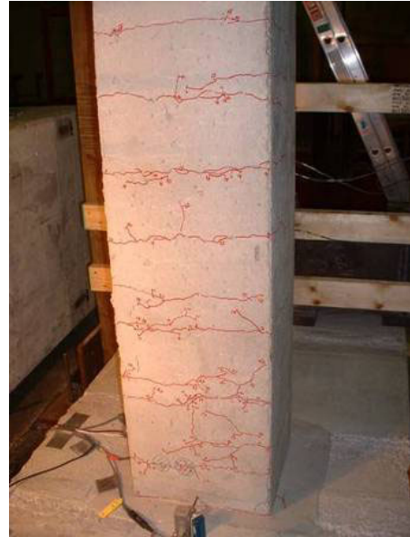
b.) East face crack progression
