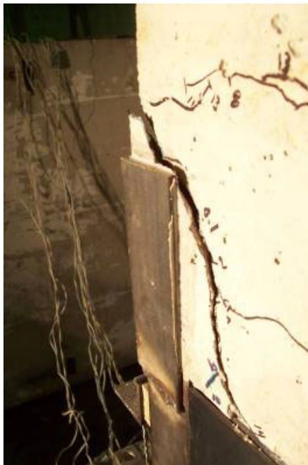
Figure 112. Photograph of Column 4 – Cycle 16a southeast retrofit angle damage.
