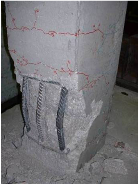
c.) Final damage to east face
