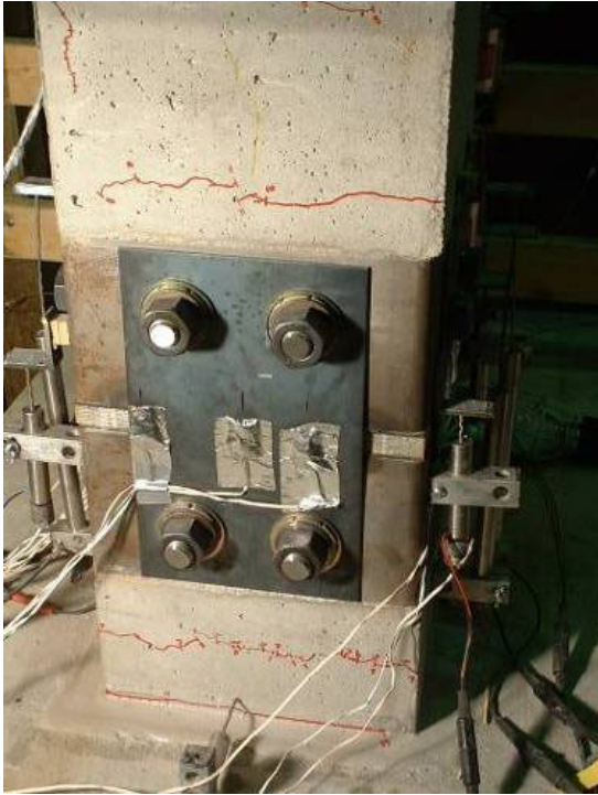
a.) Cracking around column joint
