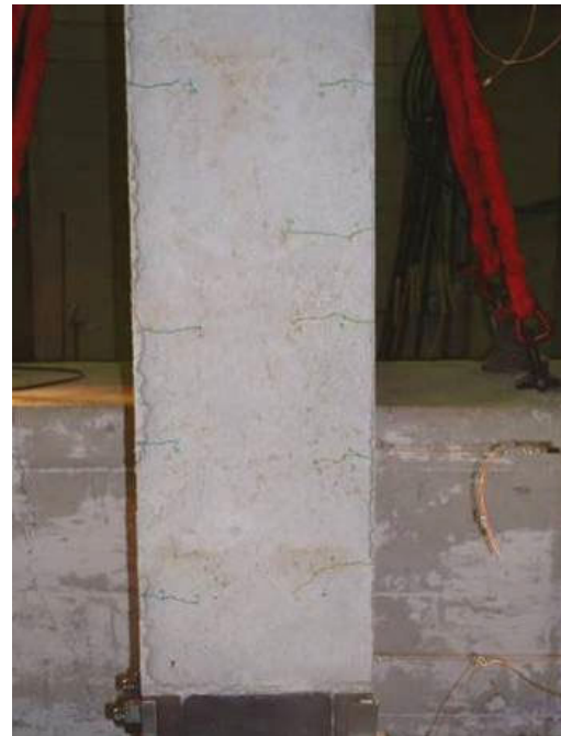
b.) North face crack progression
