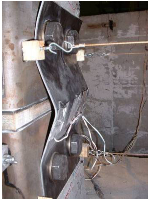
c.) West fuse plate buckling
