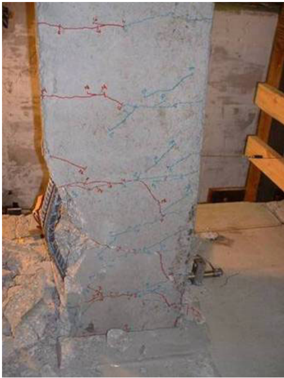
c.) North face cracking/bulging
