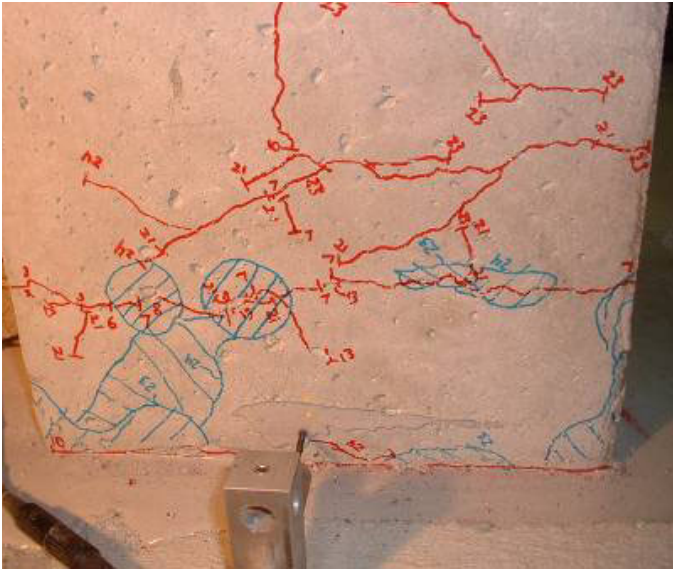
a.) East face damage
