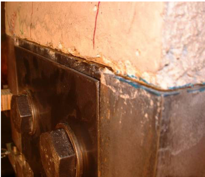
c.) West collar/column interface
