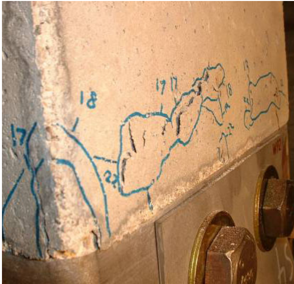
a.) Upper segment west face compression damage
