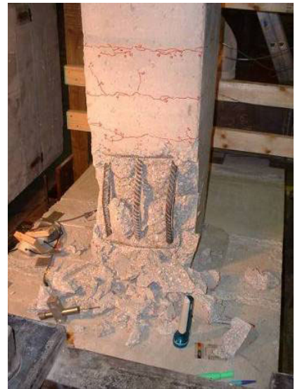
b.) East face reinforcement exposed
