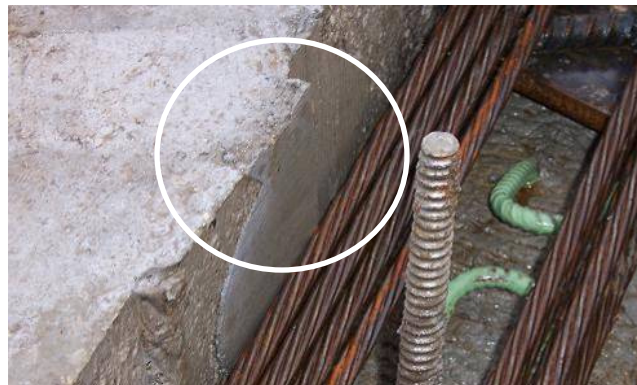
Figure 86. Concrete obstruction in Channel 1.
