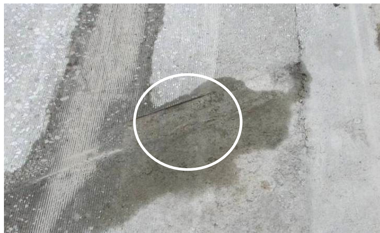
Figure 150. Low area in one transverse joint after deck grinding, December 27.
