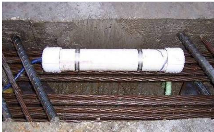
Figure 88. Vibrating wire gage with PVC pipe cover.
