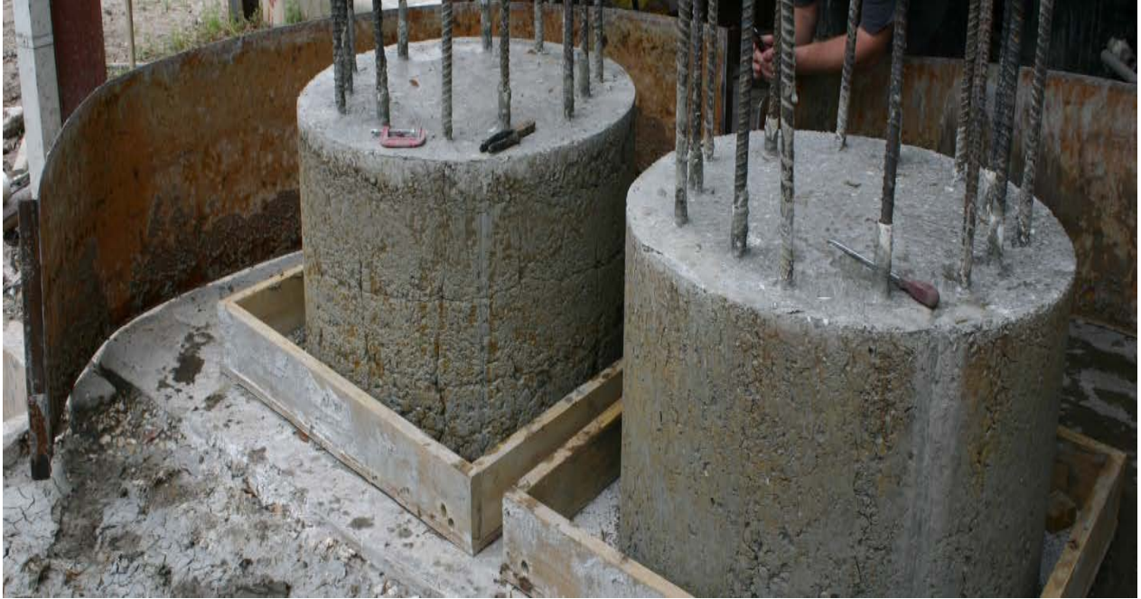
Figure 4.7. Illustrates the 90 second (left) and 40 second shaft (right) from placement one following form removal.
