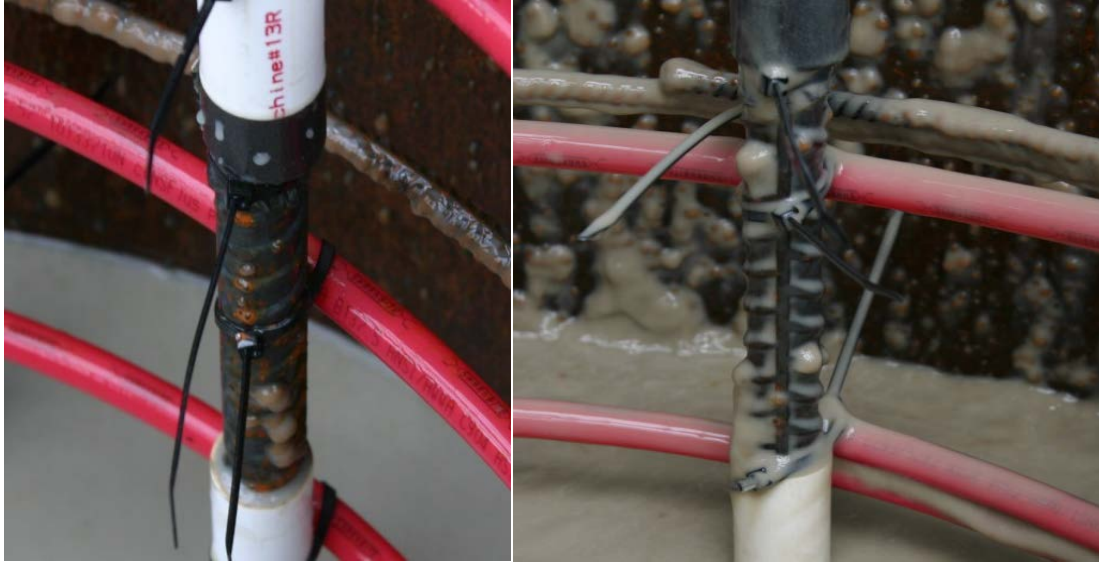
Figure 5.2. Residual slurry noticed on reinforcement 30 second (left), 50 second (right).
