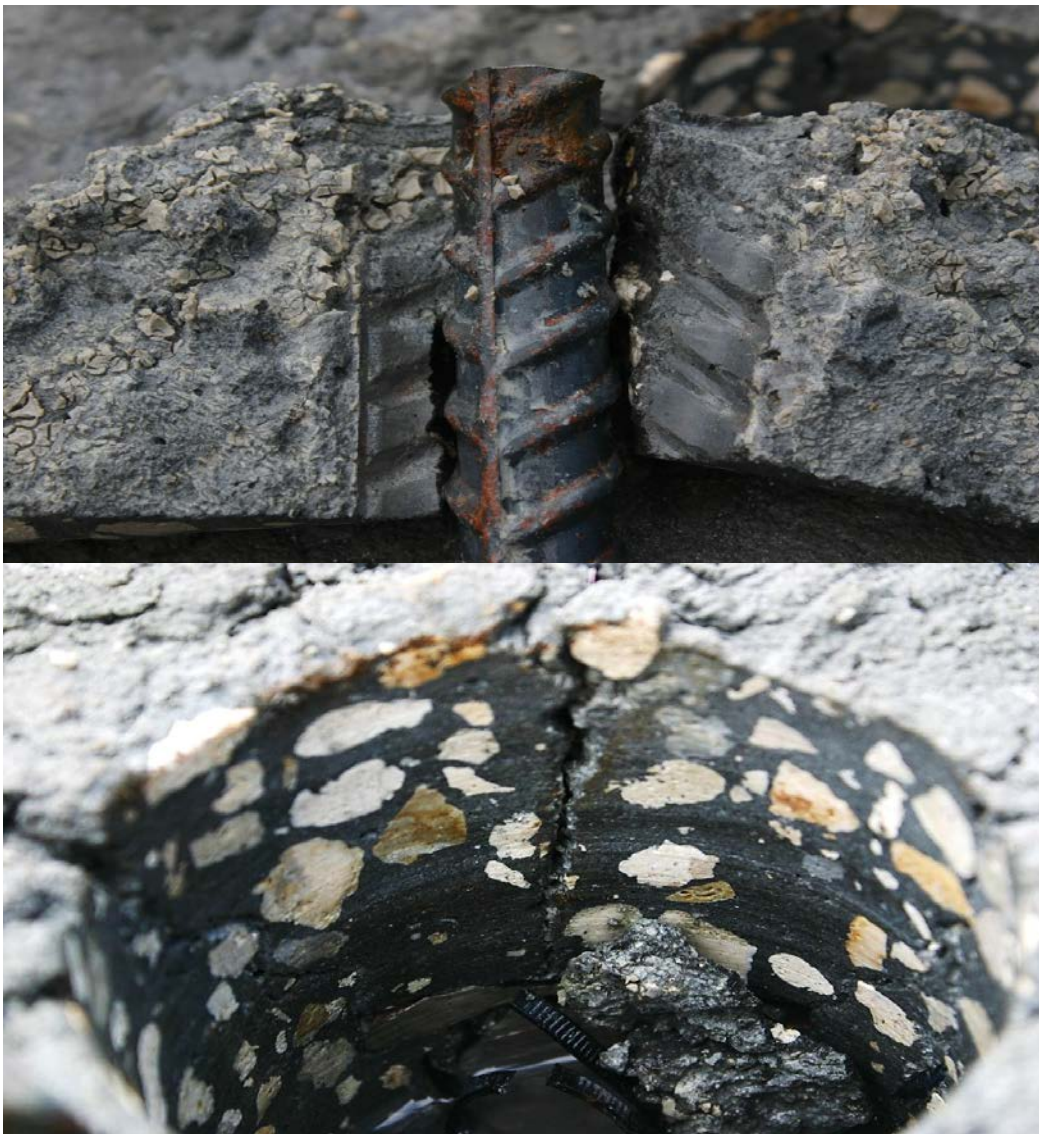
Figure 4.11. Slurry present at surface of reinforcement (top) depth of visible crease (bottom).
