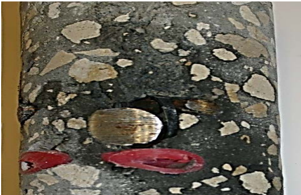
Figure 5.10. Poor consolidation around reinforcement in 40 sec/qt shaft.
