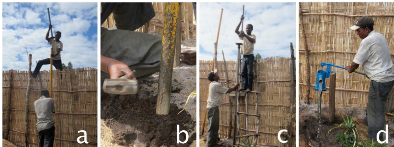
Figure 2. Typical installation of a Pompe Tany : a) percussion augering of soil; b) removed soil; c) percussion drilling of tube well/casing; d) finished pump.
