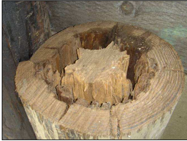
FIG. 4.6 — Internal pile deterioration that is difficult to detected using the stress wave technique
