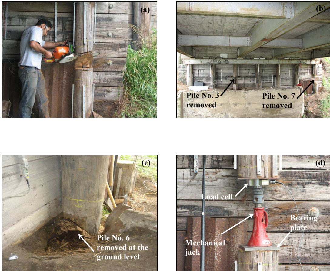
FIG. 5.7 — Destructive static load tests (a) removing pile No. 7 (b) a section from pile Nos. 3 and 7 removed (c) a section near the ground level is removed from pile No. 6 (d) mechanical jack and load cell used to restore the dead load carried by pile No. 7
