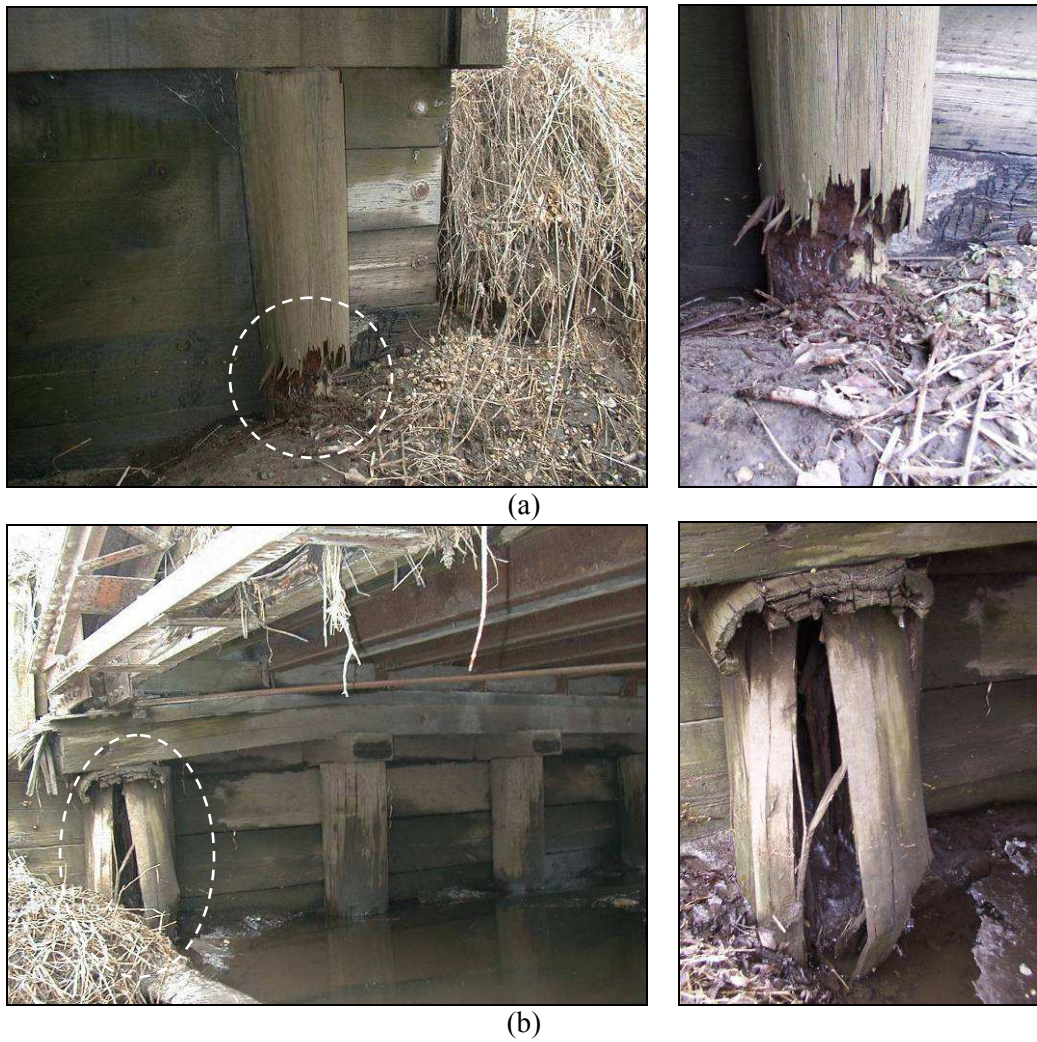
FIG. 4.1 — Timber pile biological deterioration (a) reduction of pile cross section (b) complete deterioration of pile section
