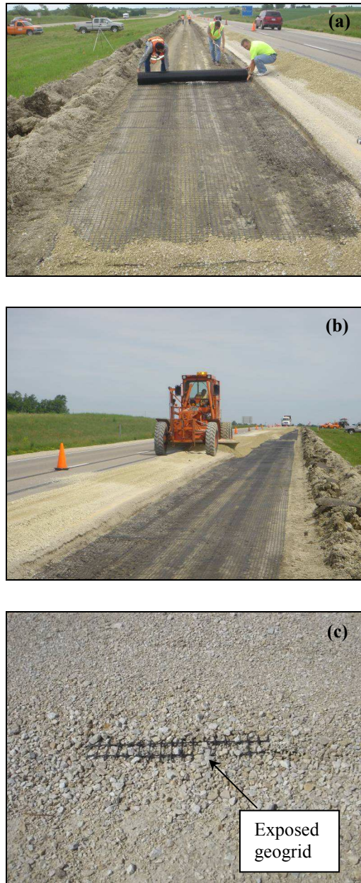
FIG. 2.15 — Geogrid stabilization (a) rolling the BX1200 geogrid over the soft subgrade layer (b) spreading crushed limestone over the geogrid (c) exposed BX1200 geogrid at about 2.4 from the pavement edge after 10 months
