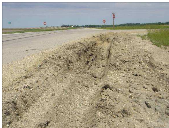
FIG. 2.14 — Severe rutting extending to the underlying clay layer
