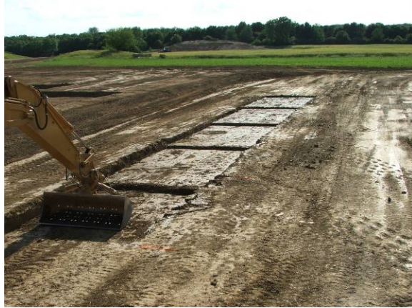
Figure 6.2. Excavation of natural subgrade for construction of Strip 2 with variable lift thickness
