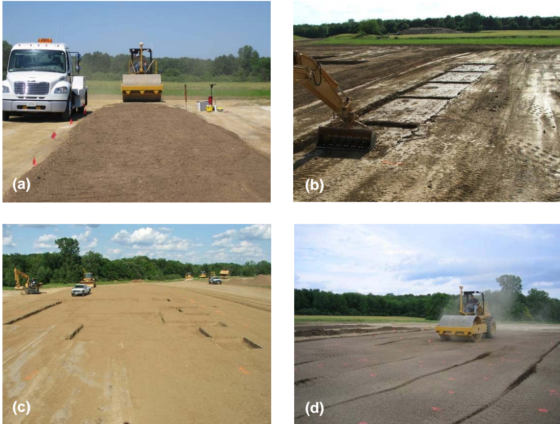
Figure 5.3. Construction and testing processes: (a) constructed test strip, (b) test Strip 1 excavations for variable lift thickness, (c) excavations for 510-mm lifts in spatial area, (d) compaction of spatial area
