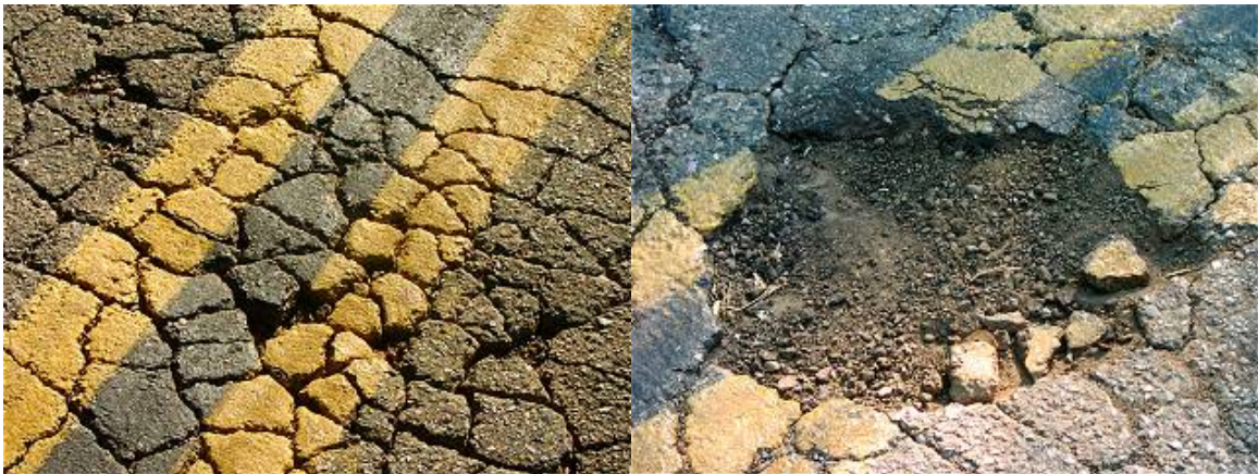
Figure 2. Alligator cracks and pothole formation
