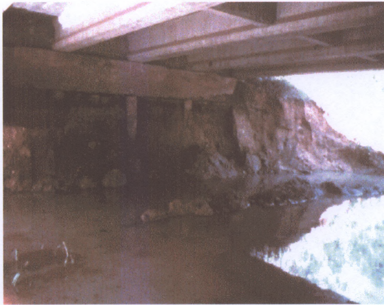
Figure 2-7 Hydraulic erosion of earth-fill embankment
