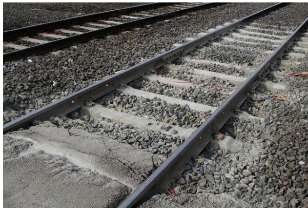
Figure 1.3 Example of Fouled Ballast
