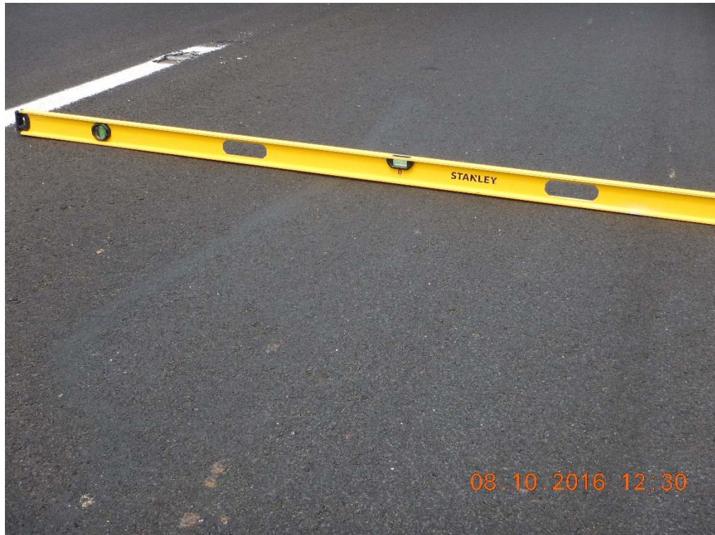
Figure 7.15: Warren-Allen County, Rutting, Fresh Microsurfacing
