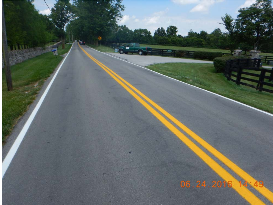
Figure 7.1: Fayette County, Bleeding Distress
