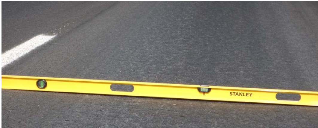
Figure 7.10: Warren County, Rutting, Microsurfacing
