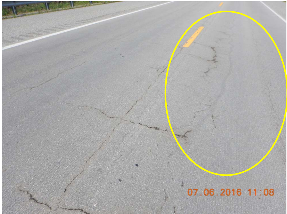
Figure 7.8: Greenup County, Alligator Cracking, Microsurfacing
