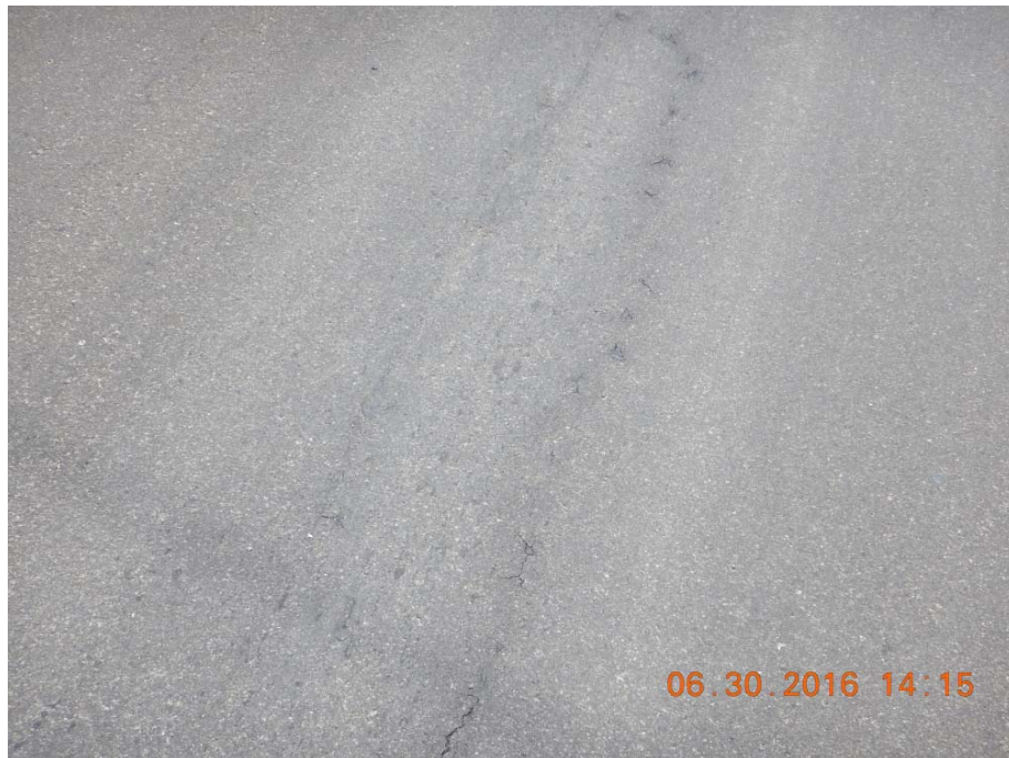
Figure 7.2: Morgan County, Bleeding Distress, Brand New Surface
