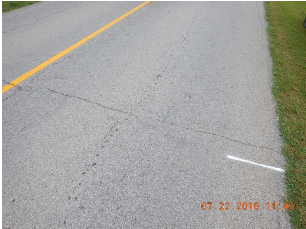
Figure 7.3: Green County, Longitudinal/Transverse Cracking, Thinlay
