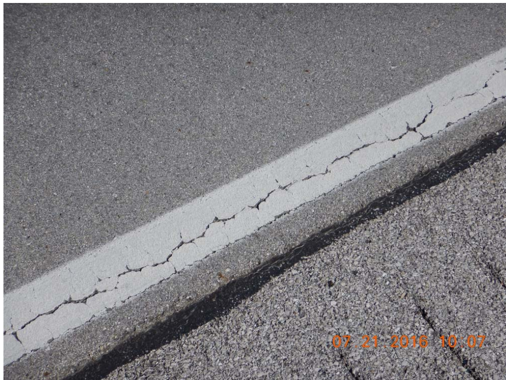
Figure 7.5: Pulaski County, Edge Cracking, Thinlay
